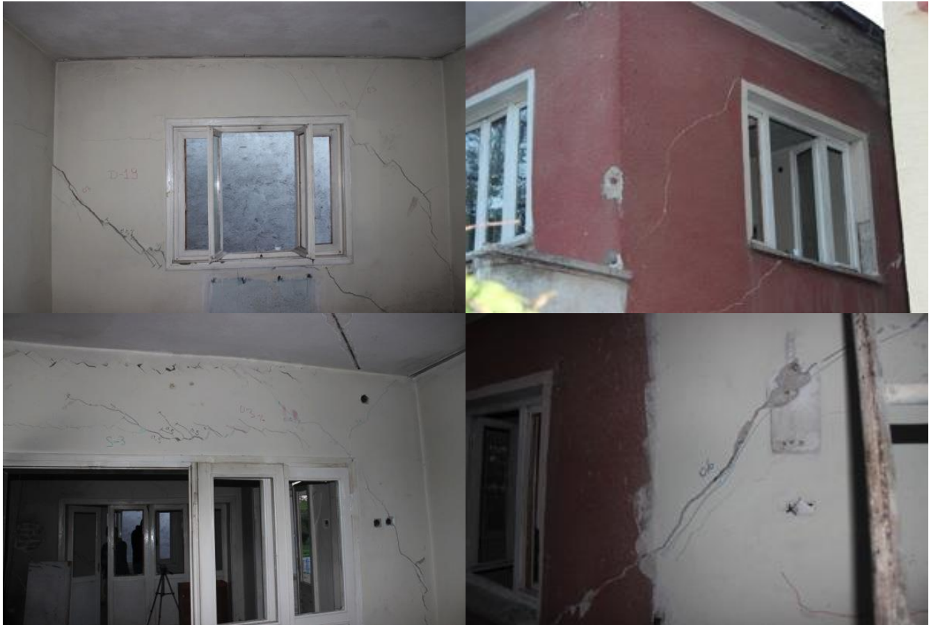
Fig. 9 – Different cracks observed during one-way cyclic test in the second story
