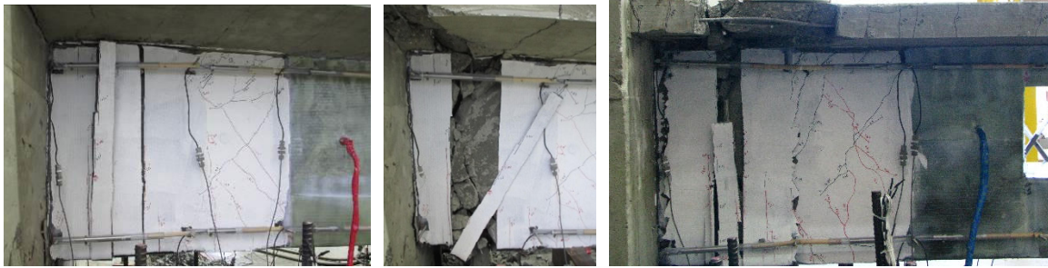
Fig. 6a, b & c – Crack patterns in specimen IA at failure region (i.e. fixed-end) at 3.0% and 4.0% drift (a & b, left & middle), and crack patterns in specimen IB at failure region (i.e. fixed-end) at 4.5% drift (c, right).
