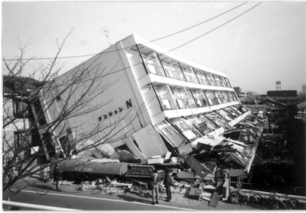
(a) Failure of a steel structure
