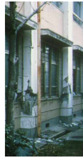
(b) Flexure-Shear failure
