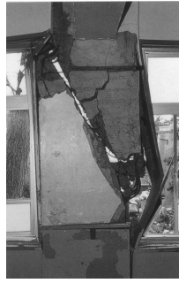
(a) Shear failure
