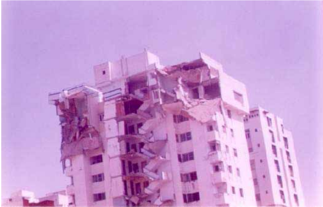
Photo No. 5 : Total Collapse Of Framed Structure At Ahmedabad (Mansi Tower)
