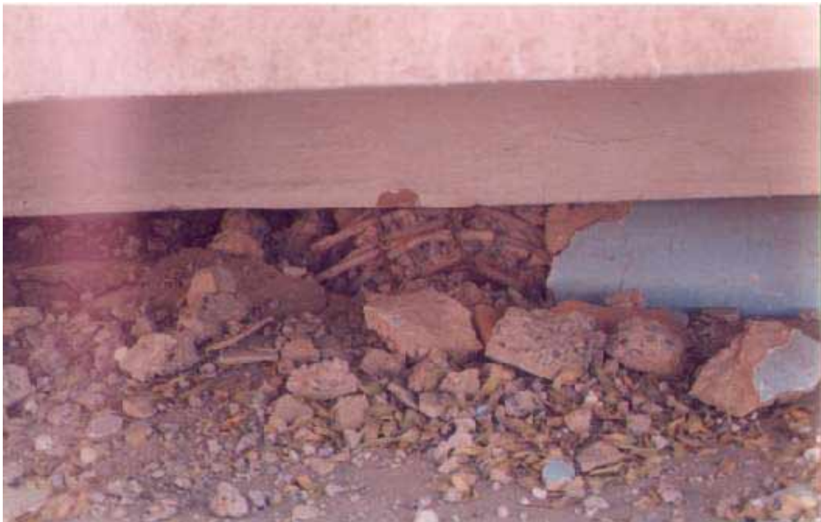
Phot No. 9 : Circular column for parking (Ground floor) after failure
