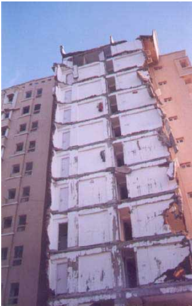
Photo No. 6 : Total Collapse Of Framed Structure At Ahmedabad (Shikhar tower)
