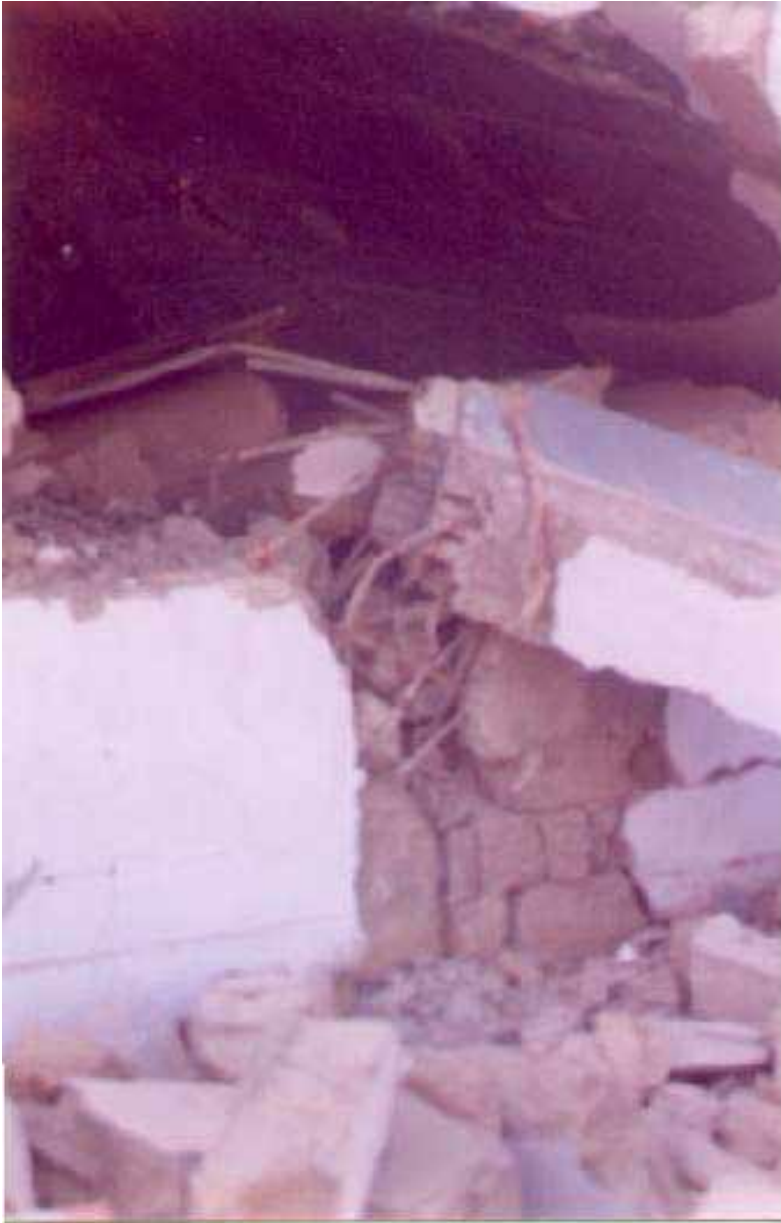
Photo No. 10 : Improper Detailing At Beam Column Joint.
