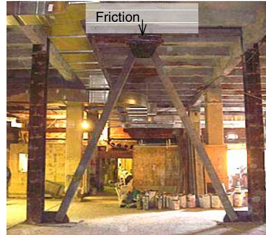
Figure 5. Friction damper at top of chevron brace.
