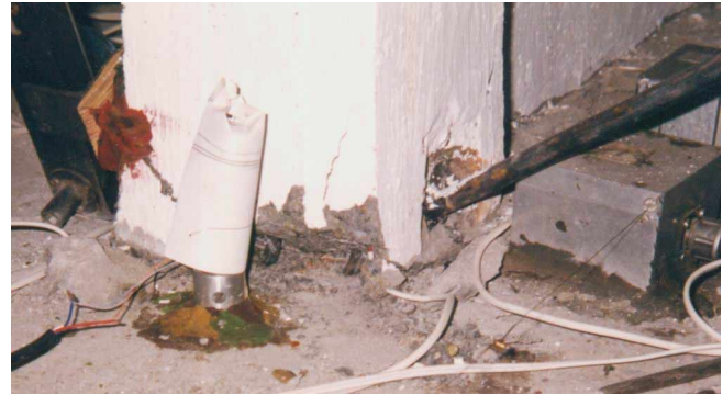
Fig. 6 Bucking of reinforcement and Crushing of concrete at the bottom of edge column of wall
