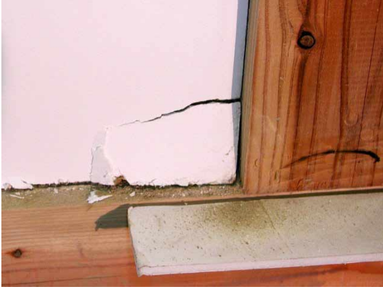
Photo 3 : [Plaster-wall test] Crack on a plaster surface.
