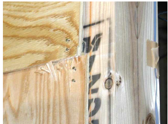
Photo 8 : [Plywood-wall test] Deterioration at corners of plywood panels.
