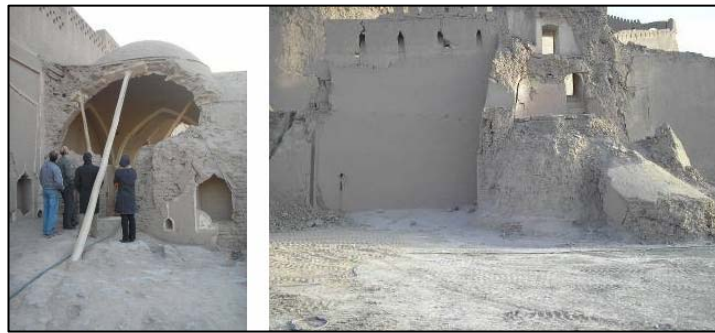
Figure 5 Disconnection between dome and walls in Stable (left) - although the First-Wall acted as a shear wall but finally the tower crashed with 45° pattern (right)
