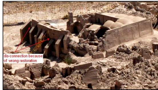
Figure 4 Incorrect interventions, the butters behind the west wall of the Caravansary
