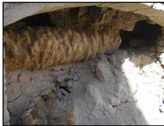
Figure 6 Termite effect on the palm tree in the wall of Ice House, Bam Citadel
