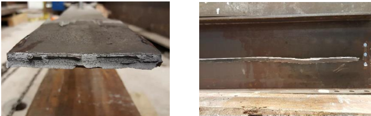
Fig. 10 Fractured Steel Plate, BRB4
