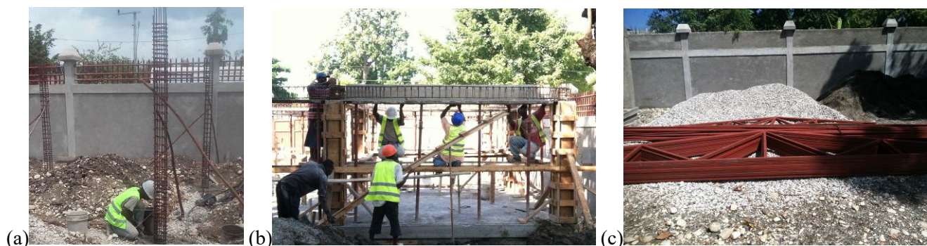
Fig. 7. (a) Standardized and prefabricated column cages being installed, (b) standardized formwork used to ensure proper column and beam sizing and spacing, (c) standardized and prefabricated roof trusses staged on site prior to installation.
