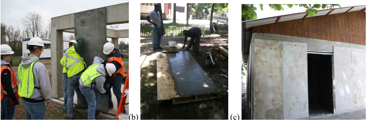
Fig. 3. (a) Concrete panel tilt-up process at the prototype built in the University of Notre Dame campus; (b) concrete panel production in Haiti and (c) first prototype structure built with concrete frame and panel system in Haiti.
