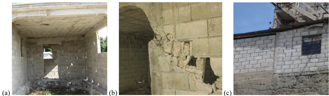
Fig. 1. Typical home in Léogâne, Haiti: (a) built with poorly confined CMU (concrete masonry unit) walls (b) typically failing in shear and bearing striking resemblance to (c) a typical CMU home in Quito, Ecuador.
