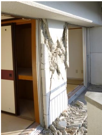
(c) Shear failure of non-structural wall
