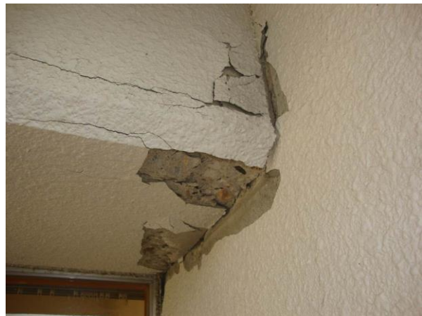
(d) Crush of concrete at plastic hinge region of a beam end
