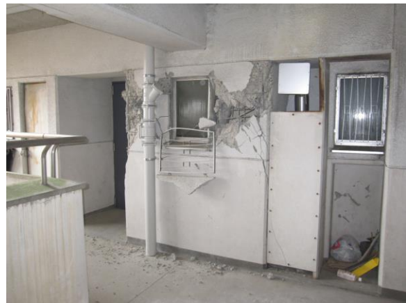
(b) Shear failure of non-structural wall
