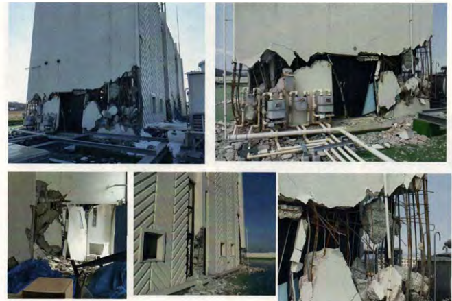
Photo 7 – Damaged pent house of a research building at Aobayama campus, Tohoku university
