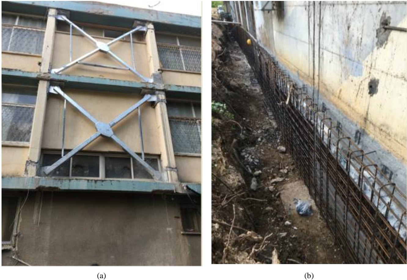
Fig. 5 – retrofit of Meginim School (Kiryat Shomna): (a) addition of yielding steel braces; (b) addition of grade-beam between foundation to reduce effects of potential ground rupture at surface level
