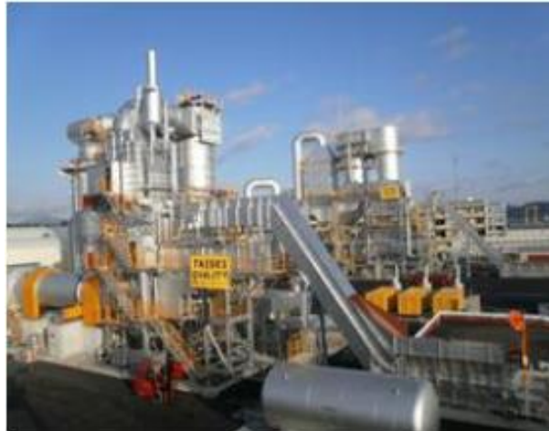
Fig. 3: Temporary incinerator in Kesenuma City, Miyagi [12].
