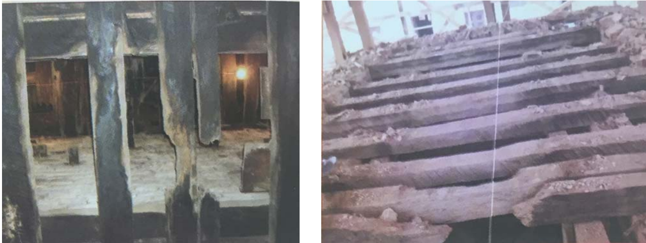
Fig. 6 – Deteriorated timber elements (before interventions) [16].
