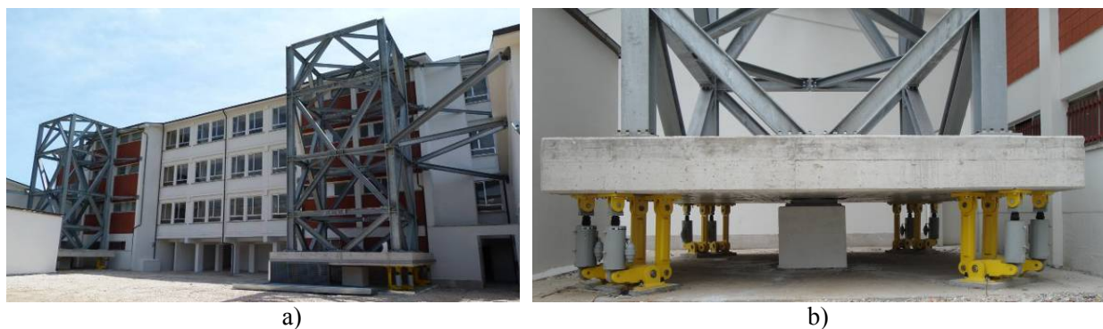
Fig. 3 - a) Building coupled with Dissipative Towers; b) Detail of the tower base: spherical hinge and viscous dampers on lever mechanisms
