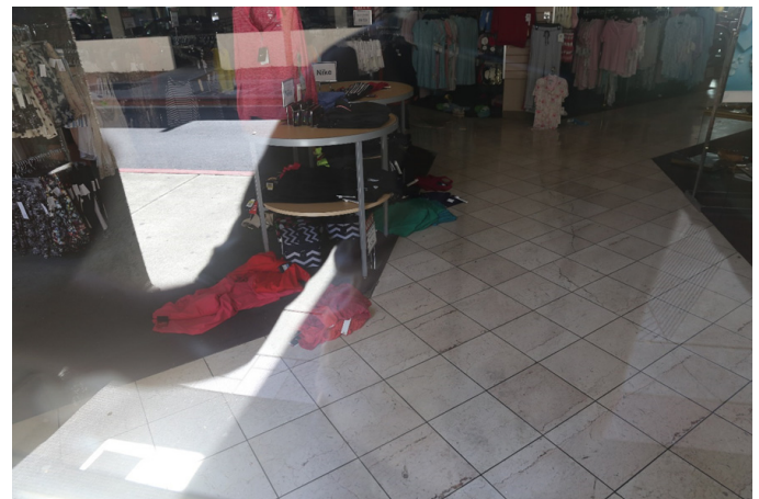
Flooded floor with merchandise on the floor
