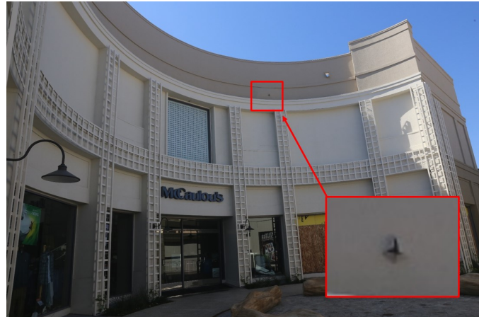
Photograph of store after water was turned off (pressure of a water head punched a hole in the parapet)
