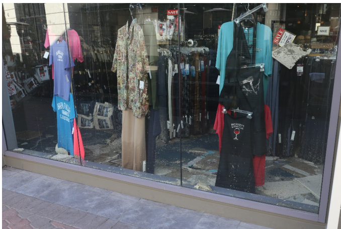
Soaked and partially dissolved lay-in panels on the floor and merchandise
