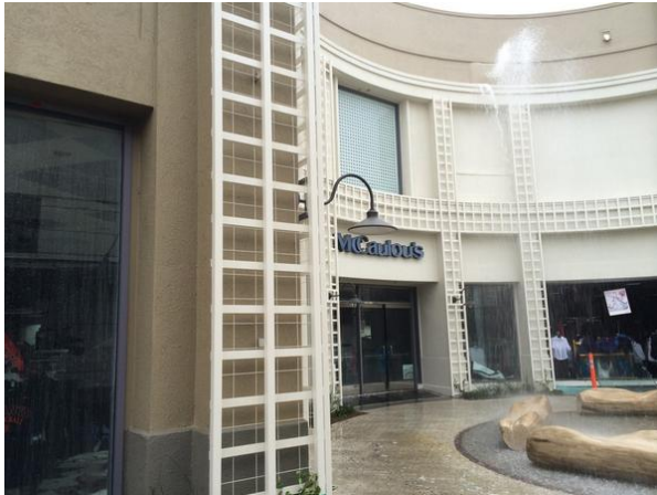
Photograph of store while water flooding was taking place
