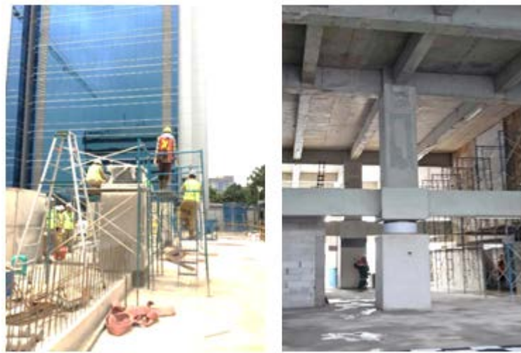
Fig. 11 Installation of S-HDRB at office tower and exhibition of the isolator to visitors
