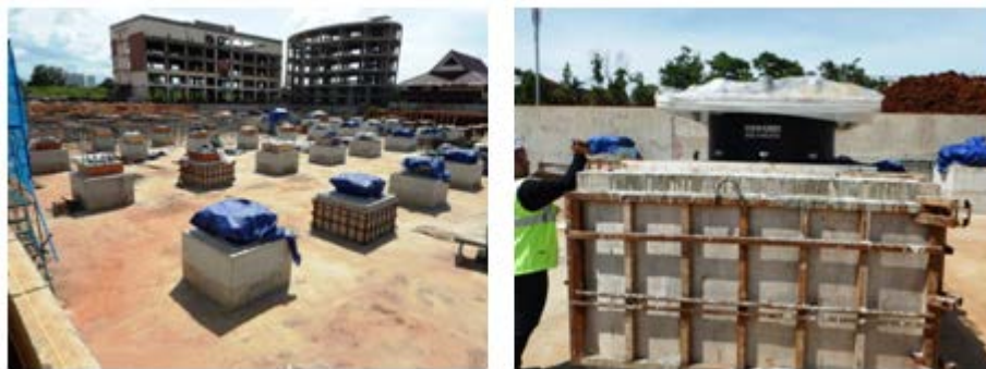
Fig. 10 Installation of S-HDRB at construction site of a hospital in Jakarta, Indonesia
