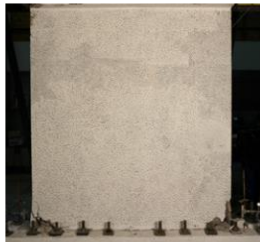
b) Sliding shear failure, WSL2
