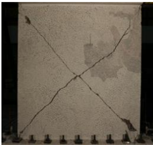
a) Brittle diagonal tension failure, WSL1
