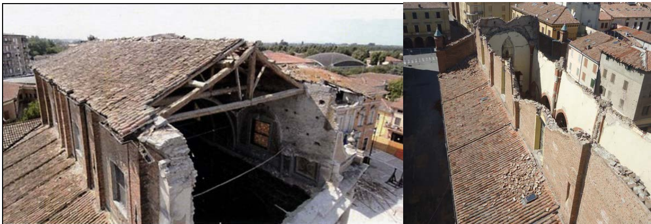
Figure 4. Partial or total collapse of roof structures in churches during the 2012 earthquake in Emilia, Italy [7].
