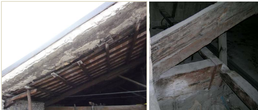
Figure 3. Results of interventions; a massive intervention over a roof truss (left) [5]; the chord of a truss was cut for unknown reasons jeopardizing safety (right)
