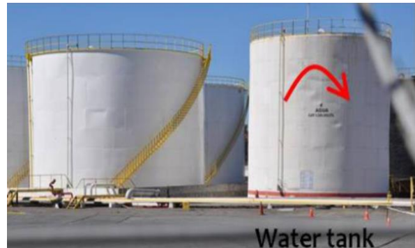
Figure 18. Tilted water tank at gas facility in the 2010 Chile earthquake.
