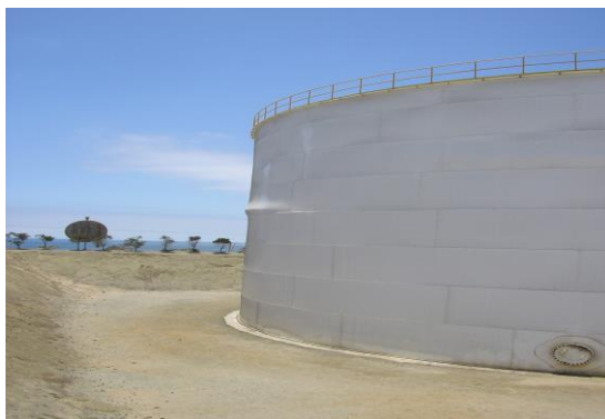
Figure 15. Tocopilla, Chile 2007 earthquake, sulfuric acid plant. Failure in the earthquake directivity.
