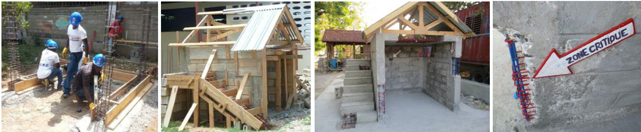
Fig. 10: a) F-Monument , b), c) with stairs, light-weight roof and concrete slab, d) critical details apparent
