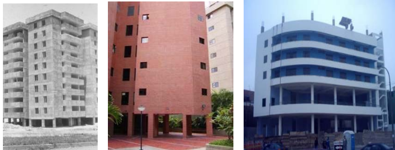
Fig.1 – Soft story in first floor [13]
