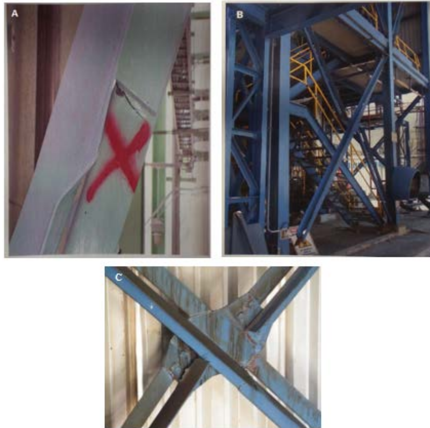
Fig. 1 – Failures observed on starred angle braces: a) Local buckling; b) Torsional buckling; c) Fracture on the cross point connection. ([4][5]).
