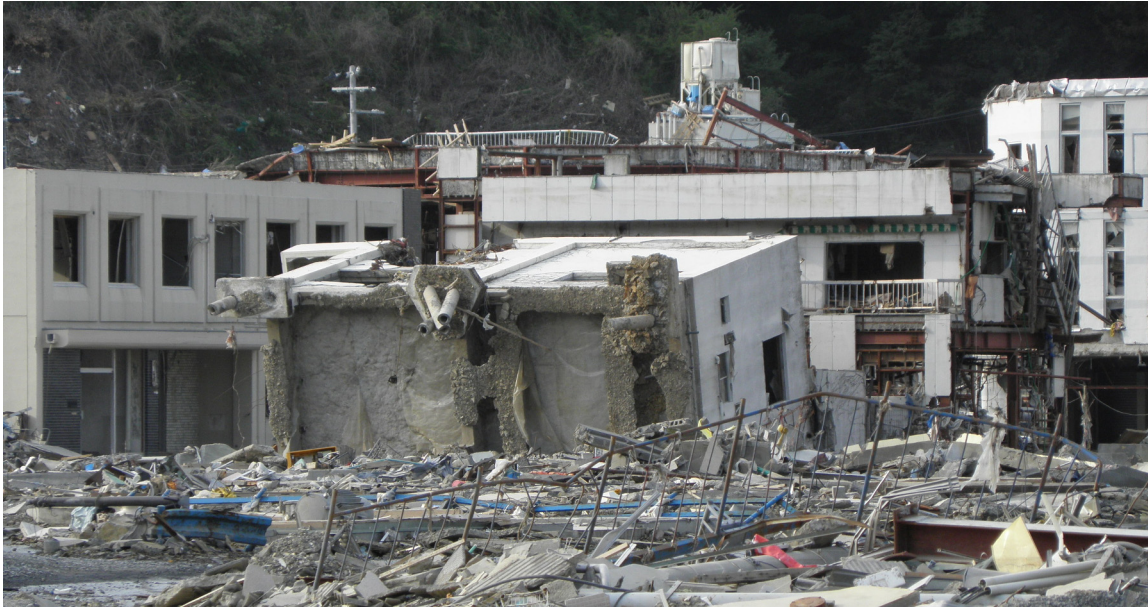
Fig. 2. Effects of uplift: overturned building in Onagawa Japan after 2011 Tohoku tsunami. Although supported by pile groups, the foundation was not sufficient to resist earthquake shaking followed by hydrodynamic and buoyancy uplift and overturning forces during the tsunami. (Photo courtesy L. Ewing).
