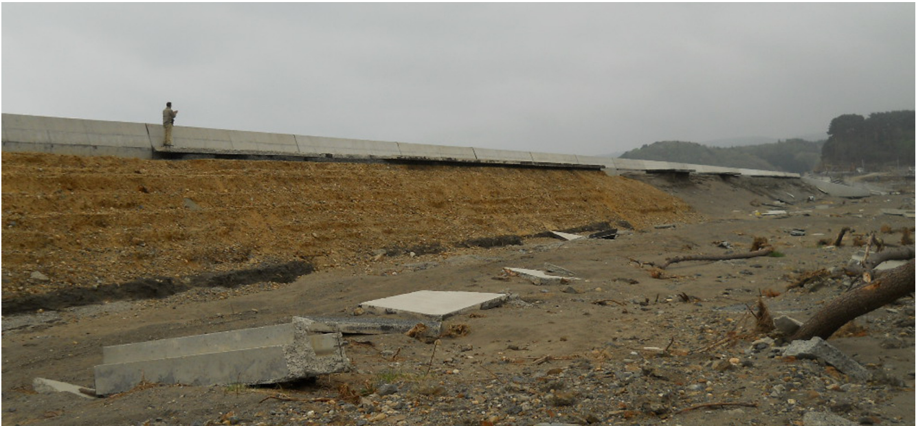
Fig. 9. Raveling of landward slope protection facing on overtopped seawall at Noda, Japan in Tohoku tsunami. Concrete panels that protected the slope are scattered in the foreground. The loss of the facing system allowed soil erosion and collapse of the seawall as seen on the right side of the photograph. (Photo courtesy B. Jones).
