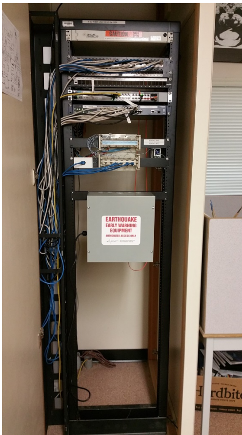
Figure 4a. System control and alarm box
