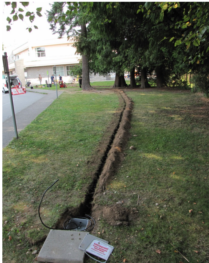
Figure 4b. Surface junction box and trench
