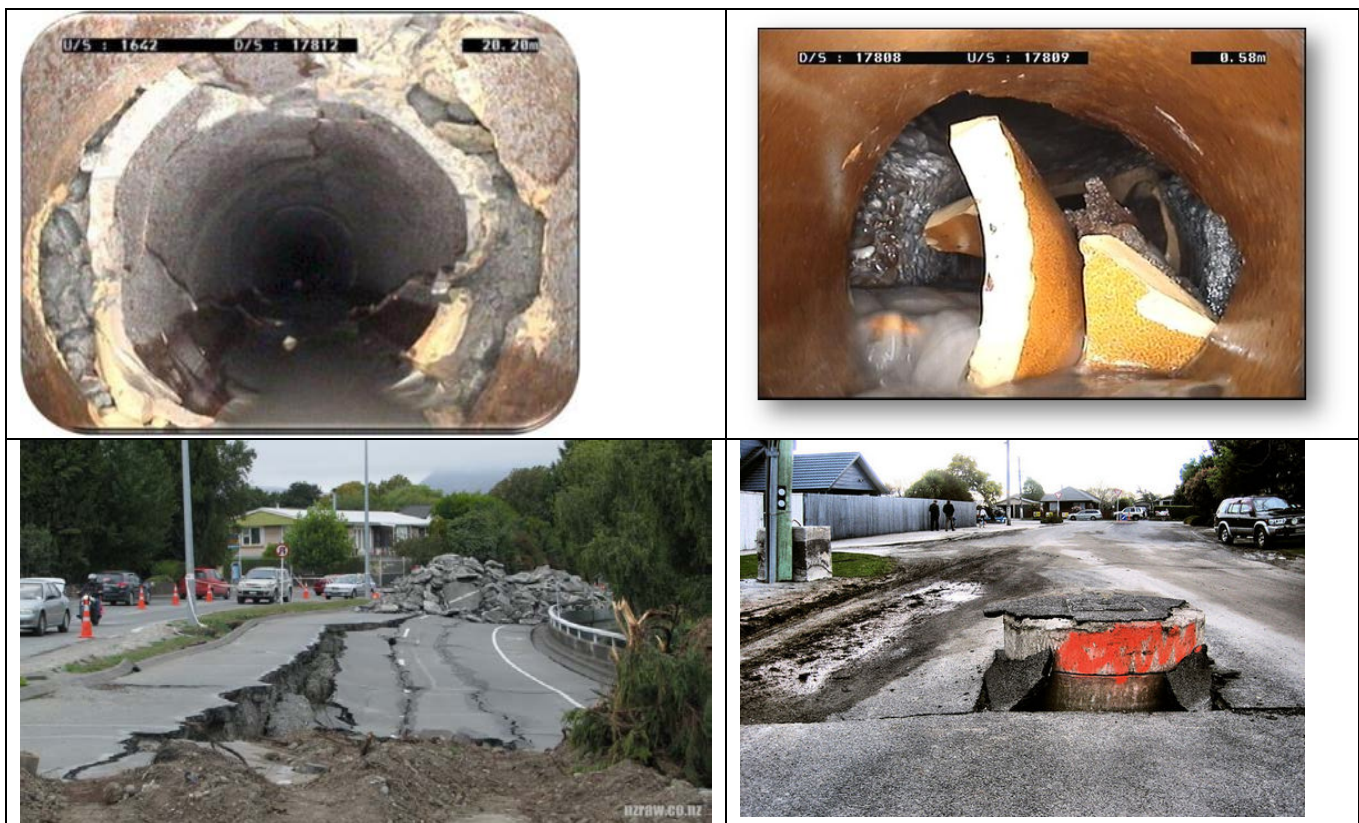
Figure 5: Sample photos of earthquake damage photos appear courtesy of SCIRT
