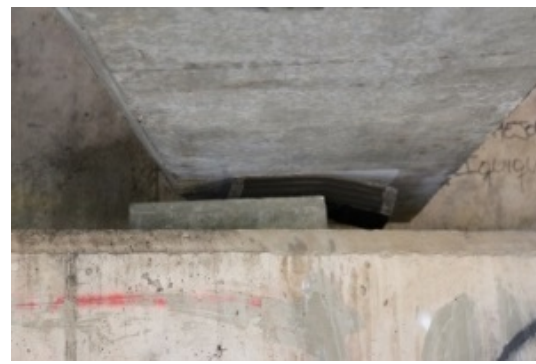
d) Sliding of elastomeric bearing, Talinay underpass, 2015 Illapel earthquake
