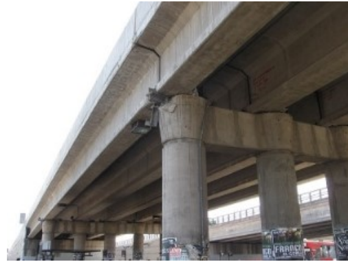
b) Transverse displacement of superstructure, Independencia overpass, 2010 Maule earthquake
