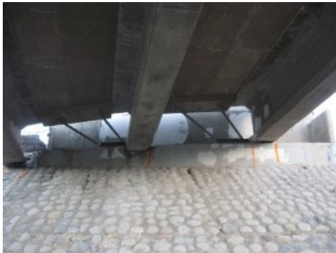
c) Transverse displacement of superstructure and deformed seismic bars, Las Mercedes underpass, 2010 Maule earthquake
