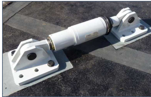
Fig. 12 – Installed shock absorber
