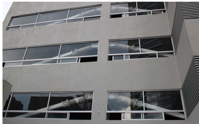
Fig. 14 – SA installed in the Lerma 256 building
