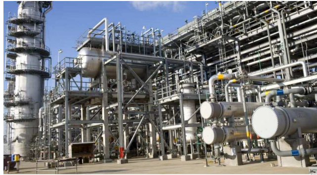
Fig. 10 – Oil refinery area equipped with elastomeric isolators
