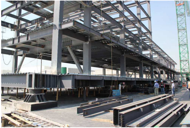
Fig. 5 – Isolators at the base of the Hotel Via Vallejo building during construction
