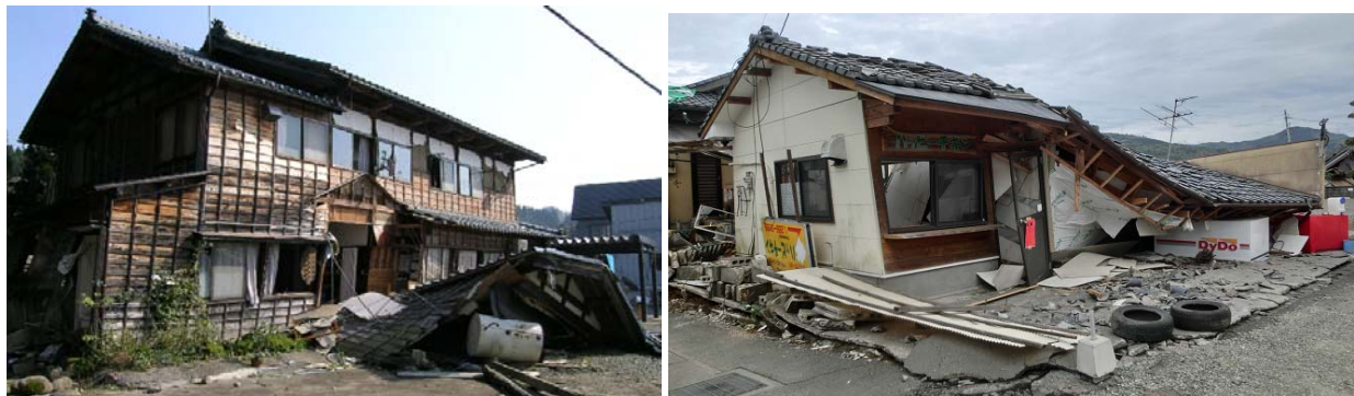
(a) 2004 Chuetsu Earthquake (b) 2016 Kumamoto Earthquake Photo 2 – Partial Collapse of wood houses
