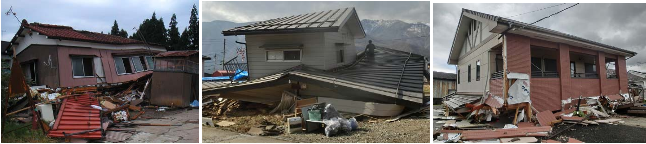
(a) 2004 Chuetsu Earthquake (b) 2014 Kamishiro Fault Earthquake (c) 2016 Kumamoto Earthquake Photo 1 – Collapsed wood houses
