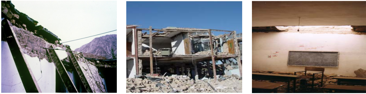
Fig. 5- Collapse of jack arch slabs (partial and complete) for lack of integrity
