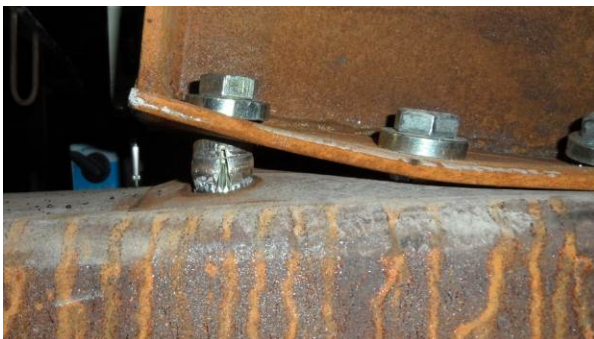
Fig.14 – Blind bolts pulled out from the column
