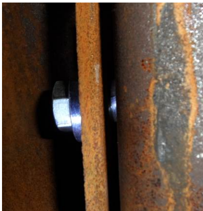
Fig.10 – The end plate separating from the column wall
