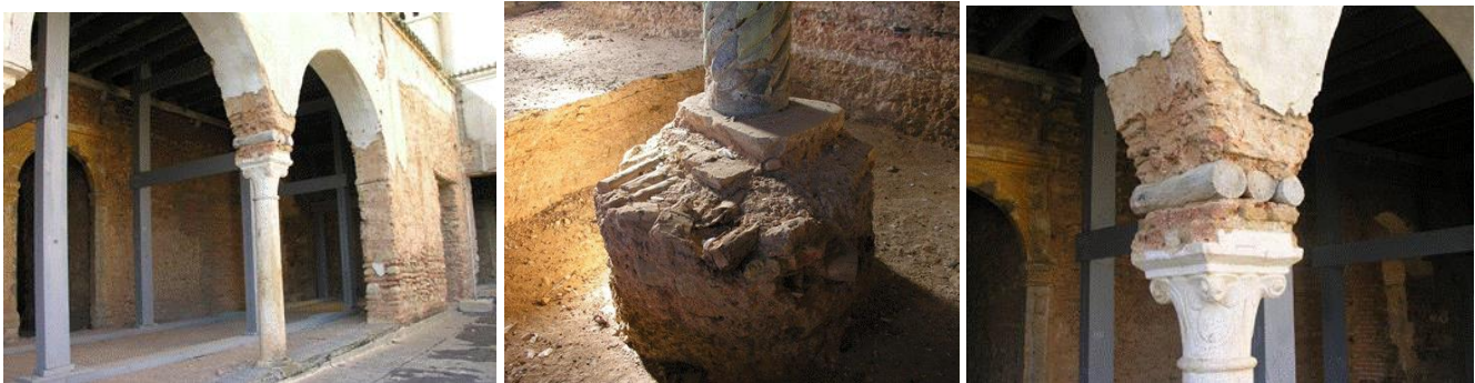
Fig. 11 – Timber reinforcements after the 1716 Algiers earthquake (P. Clemente – ENEA)
