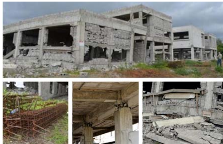
Fig. 6 – Collapse of Jama School (new building under construction)
