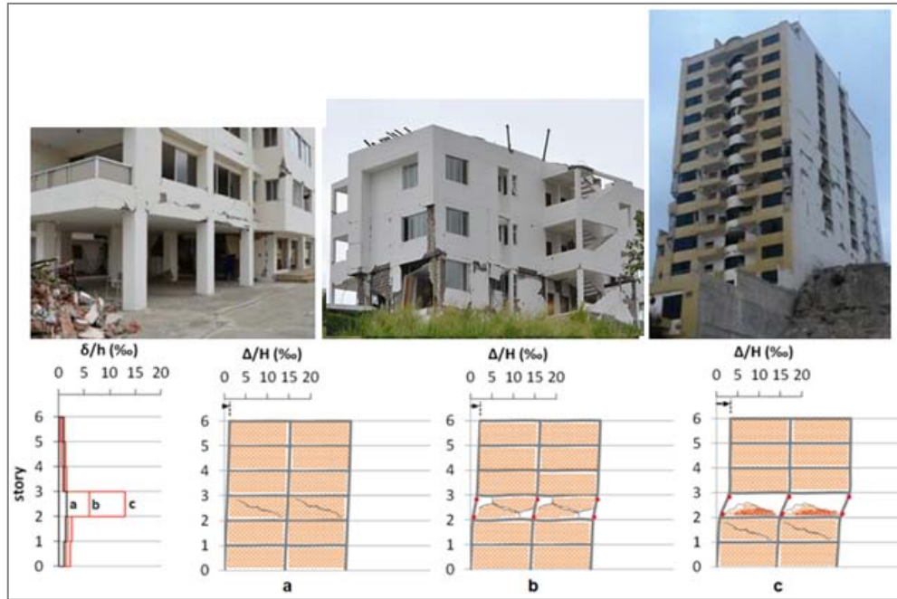
Fig. 5 – Soft/weak story performance
