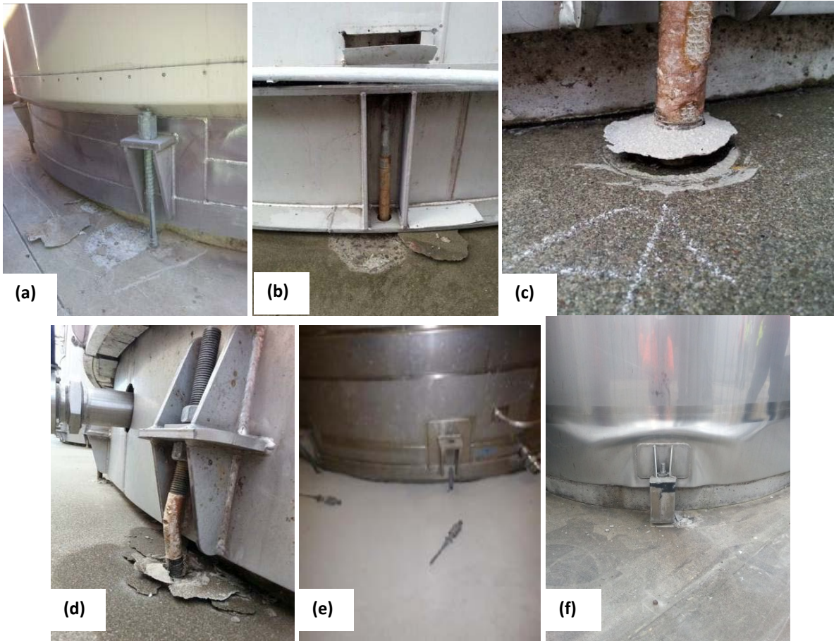
Anchorage failure by pullout, bolt tensile fracture and bolt shear failure
