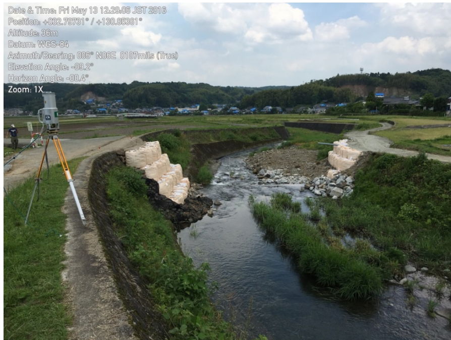
Fig.7 The terrestrial LiDAR setup and damage to the canal embankments. The main fault crossing is at the location of the repairs visible in the photograph.
