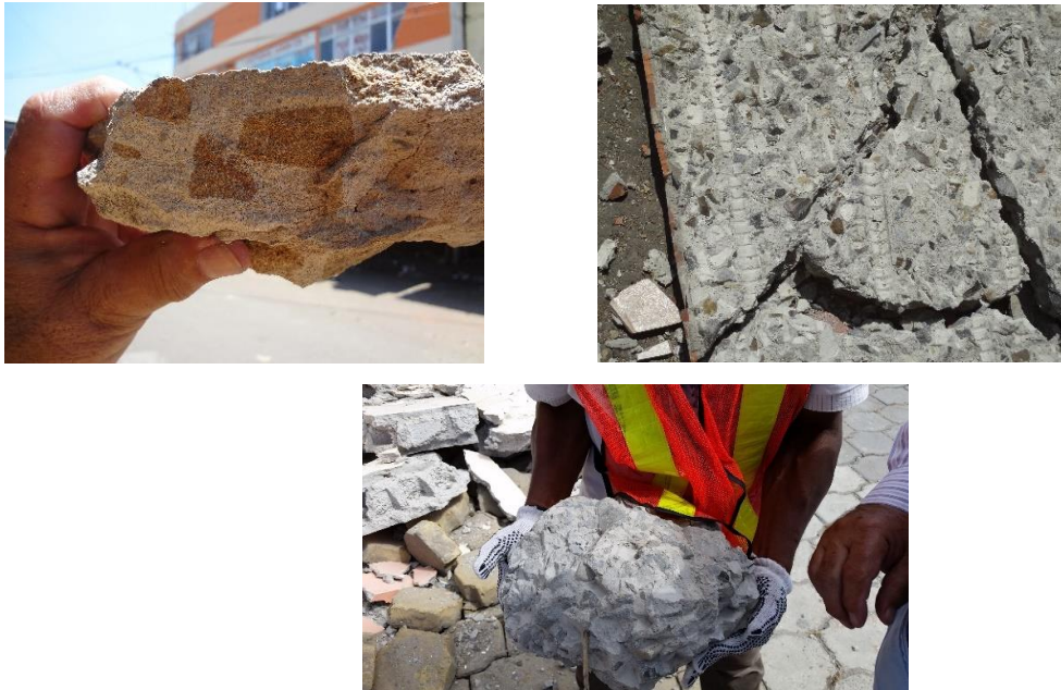
Fig. 7 – Characteristics of concrete in damaged and collapsed structures. (Up-left) Large coarse aggregate with high segregation and large amount of mortar. (Up-right) Detached concrete coating with low amount of mortar, showing very low or lack of adherence with steel deformed bars. (Down) Large amount of coarse aggregate with very few mortar
