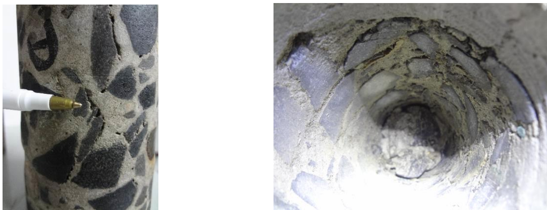
Fig. 10 – Mylonitization of coarse aggregate in concrete core samples before testing (left). Mylonitization effect inside a structural column after core extraction, showing tremendous impact in concrete integrity (right)
