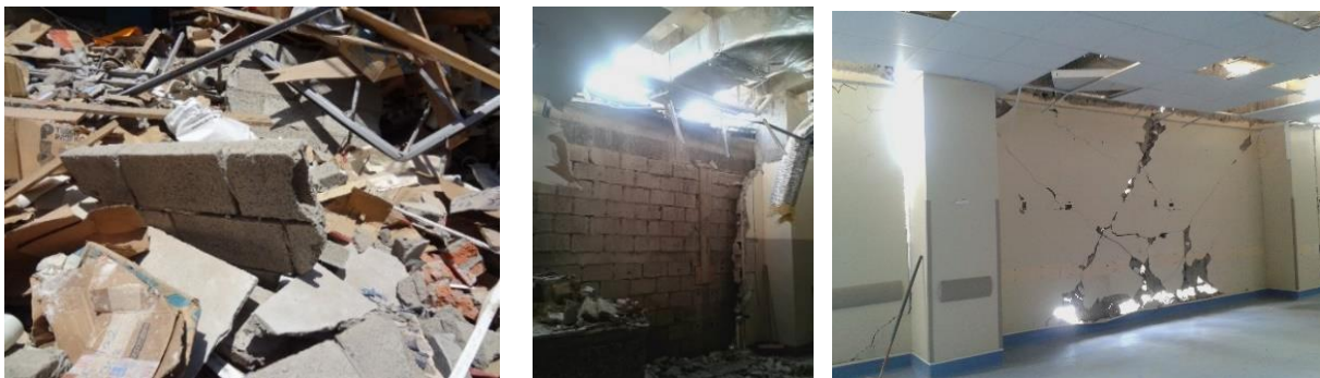
Fig. 12 – Characteristics of concrete block units used for masonry walls. Thin masonry walls with incomplete mortar handwork between units and very long and high masonry panels without bracing system.
