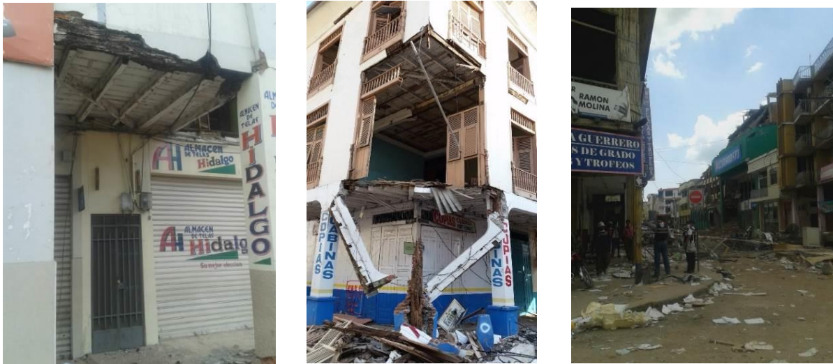
Fig. 4 – Grade of deterioration of wooden elements discovered after earthquake. Perhaps, service life ended before the quake
