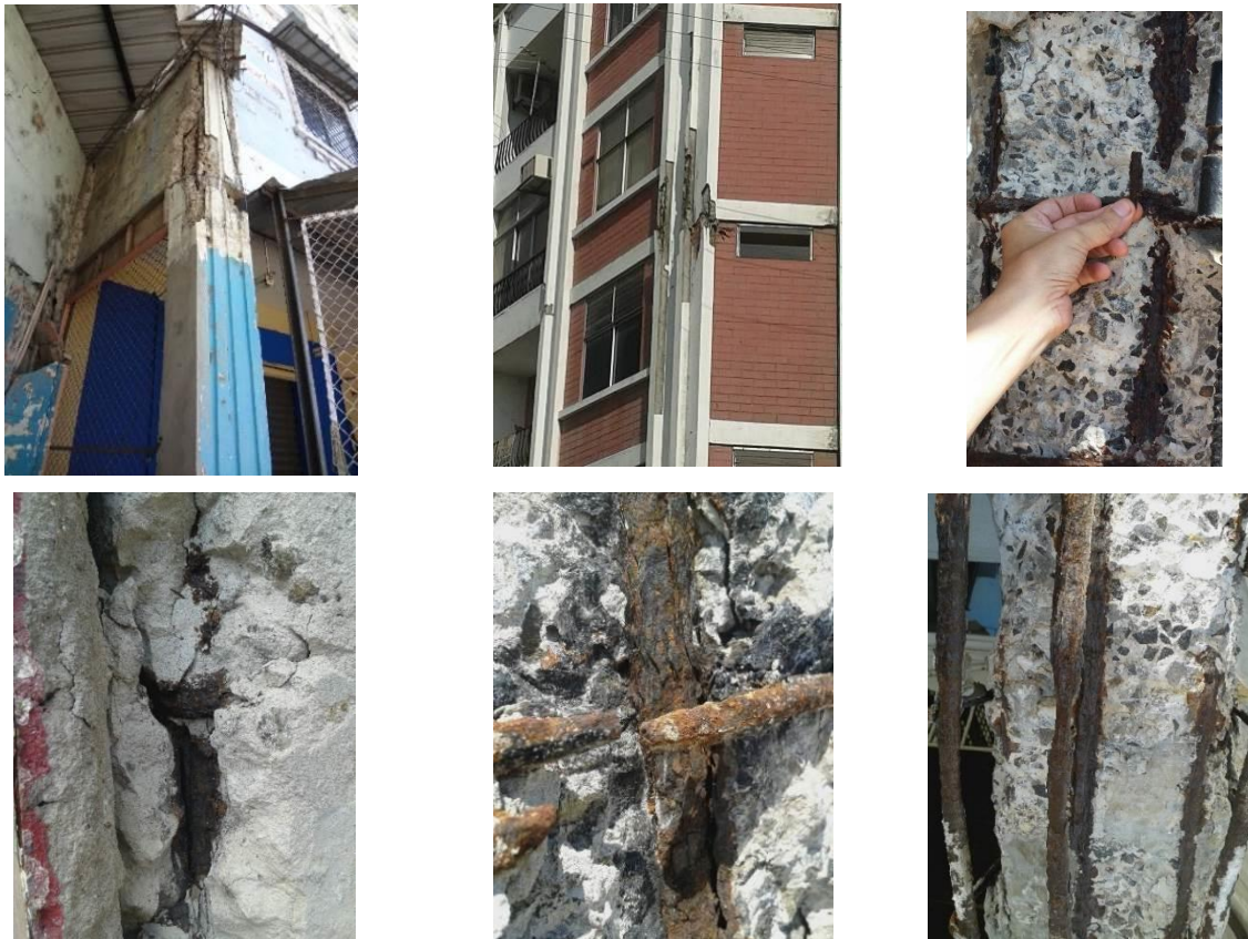
Fig. 8 – Strong corrosion in steel reinforcement (deformed and smooth bars) in old and new structures. Column steel bars can be destroyed completely using hand fingers
