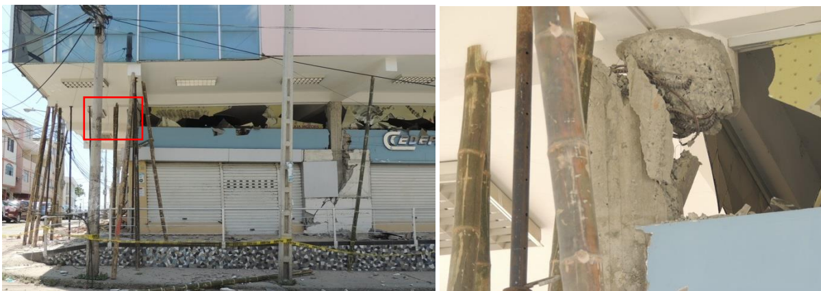
Fig. 11: Plastic hinges formed in the first floor columns of this building in Manta (GPS coordinates: 0^{\circ}57'9.5''S , 80^{\circ}42'49.4''W ). (Photos by C. Arteta Torrents)
