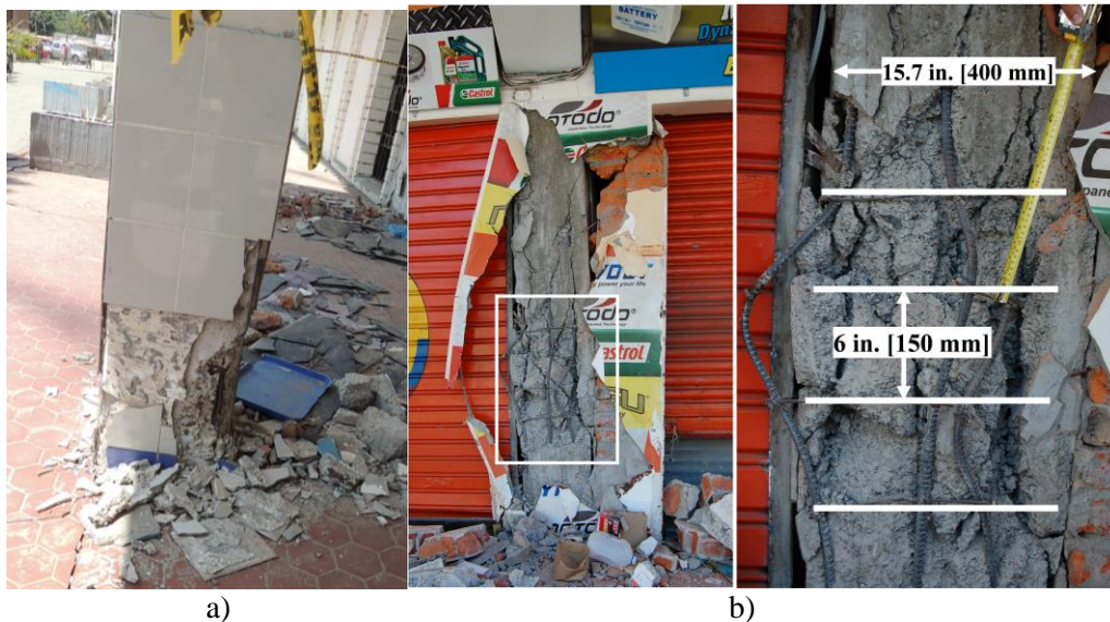
Fig. 5: a) A first floor column in the three-story Hotel Las Gaviotas in Tarqui, Manta. There is significant spalling which can be attributed to both previously corroded steel and the seismic demand imposed by the earthquake (GPS coordinates: 0°57'5.7"S, 80°42'48.5"W). b) Small-diameter-hoop spacing details of a first floor unconfined column in a four-story commercial building in Tarqui, Manta (GPS coordinates: 0°57'14.9"S, 80°42'53.9"W). (Photos by C. Arteta Torrents)
