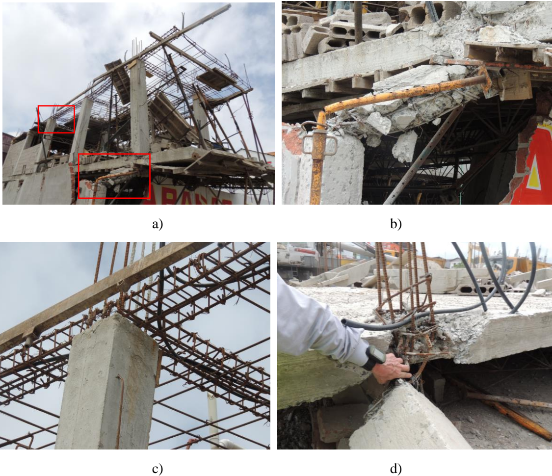
Fig. 7: a) & b) Failure of first floor columns in a building under construction in Canoa. The column has large stirrup spacing. c) The slab to column connection at the edge shows a lack of dowels and therefore provides no structural integrity (GPS coordinates: 0°27'42.67"S, 80°27'20.67"W) (Photos by GMSLLP & C. Arteta Torrents) d) Failure of first floor columns in building under construction in Canoa. The slab to column connection at the edge shows a lack of dowels and therefore provides no structural integrity (GPS coordinates: 0°27'42.67"S, 80°27'20.67"W) (Photos by GMSLLP)
