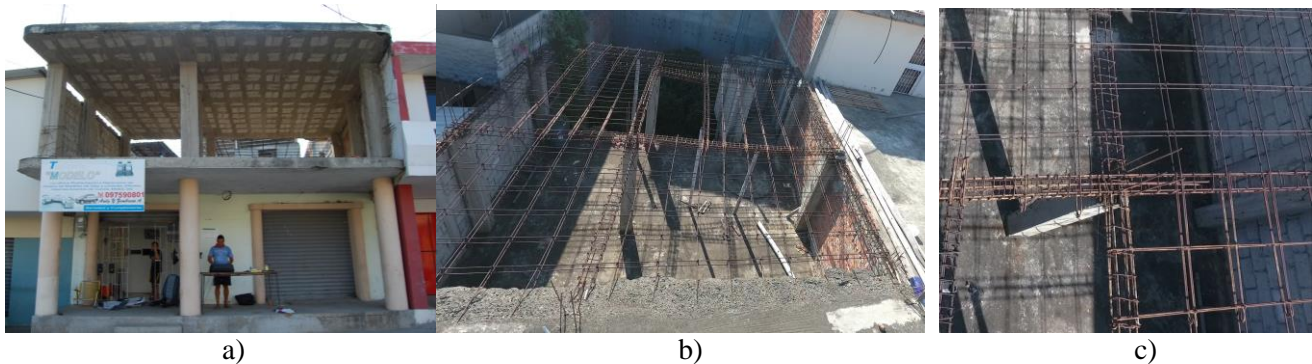
Fig. 3: a) Residential building under construction with two-way waffle slabs in Tarqui, Manta. (GPS coordinates: 0°57'28.67"S, 80°42'32.41"W). b & c) Details of beam reinforcement near a beam-column joint in the back of the house (GPS coordinates: 0°57'28.67"S, 80°42'32.41"W). (Photos by GMSLLP & Droneando ©)
