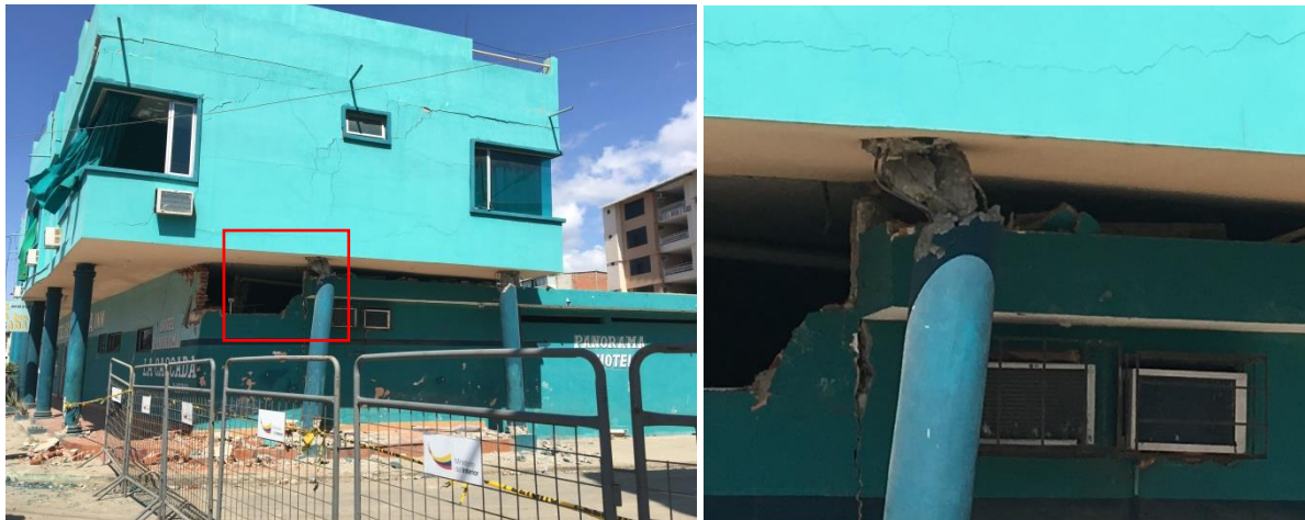
Fig. 10: Plastic hinging in the first floor columns of this residential building with first floor commercial occupancy in Tarquí, Manta (GPS coordinates: 0^{\circ}57'7.1''S , 80^{\circ}42'55.3''W ).
