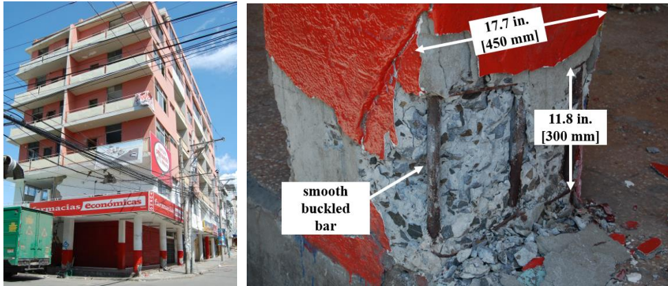
Fig. 6: Damage at the base of six-story mixed-occupancy building in Tarqui, Manta. There is significant spalling at the bottom of the first floor columns, exposing smooth longitudinal rebar and hoop spacing of approximately 2/3 of the column width. (GPS coordinates: 0°57'14.55"S, 80°42'53"W). (Photos by C. Arteta Torrents)
