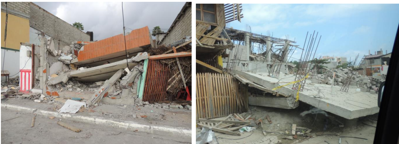
Fig. 19: a) Collapse of building with flat slab construction in Pedernales (GPS coordinates: 0°4'2.5"N, 80°3'33.9"W) (Photo by GMSLLP). b. Collapsed building that was under construction. The construction type was reinforced concrete two-way flat slabs supported on columns (GPS coordinates: 0°27'43.8"S, 80°27'21.0"W). (Photos by GMSLLP)
