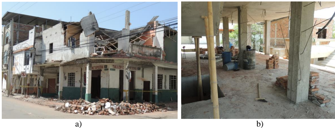
Fig. 17: a. Residential building in Tarqui, Manta, where the exterior walls collapsed. The roof also fell in this property. (GPS coordinates: 0°57'14.6"S, 80°42'38.5"W). (Photos by GMSLLP). b. This is a site of new construction. These are dowels at the concrete columns to be attached to the nonstructural walls (GPS coordinates: 0°57'7.31"S, 80°42'26.44"W). (Photo by GMSLLP)
