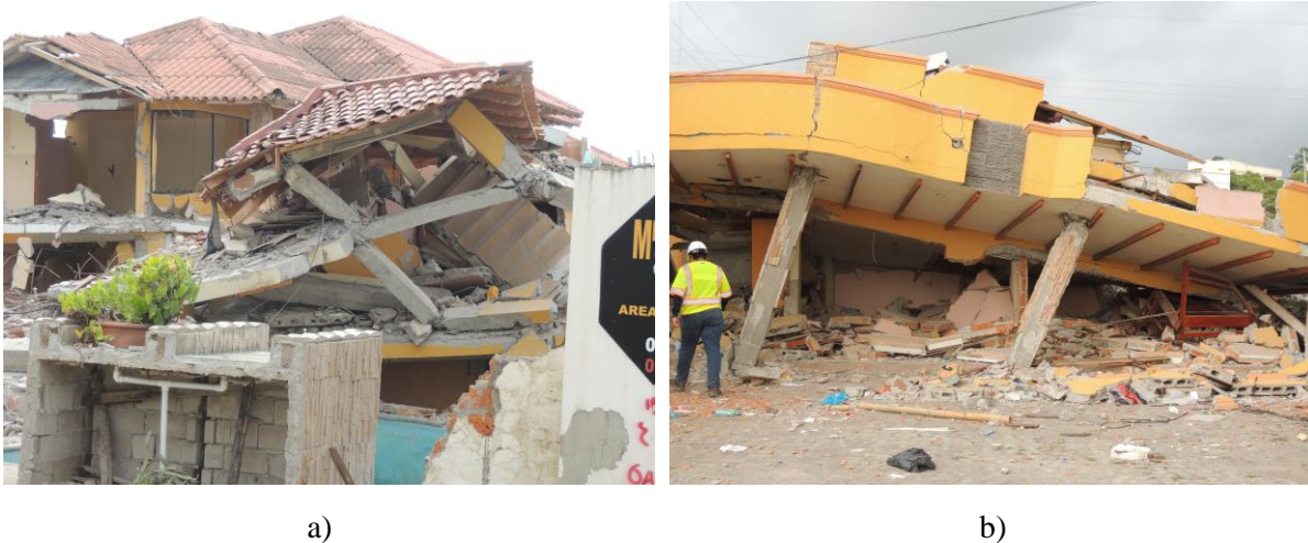
Fig. 18: a) Sideway collapse of residential structure in Pedernales (GPS coordinates: 0°4'4.8"N, 80°3'23.5"W). (Photo by GMSLLP) b) Building collapse in Pedernales. The columns shown have hinges at both ends (GPS coordinates: 0°4'3.94"N, 80°3'24.6"W) (Photo by Photos by GMSLLP)
