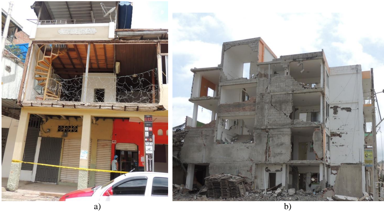
Fig. 16: a) Concrete building with wood and metal deck extension in Portoviejo. Nonstructural wall completely collapsed (GPS coordinates: 0°57'14.6"S, 80°42'38.5"W). b) Concrete building in Canoa where brick and masonry exterior walls collapsed. (GPS coordinates: 0°27'46.59"S, 80°27'23.56"W). (Photos by GMSLLP)
