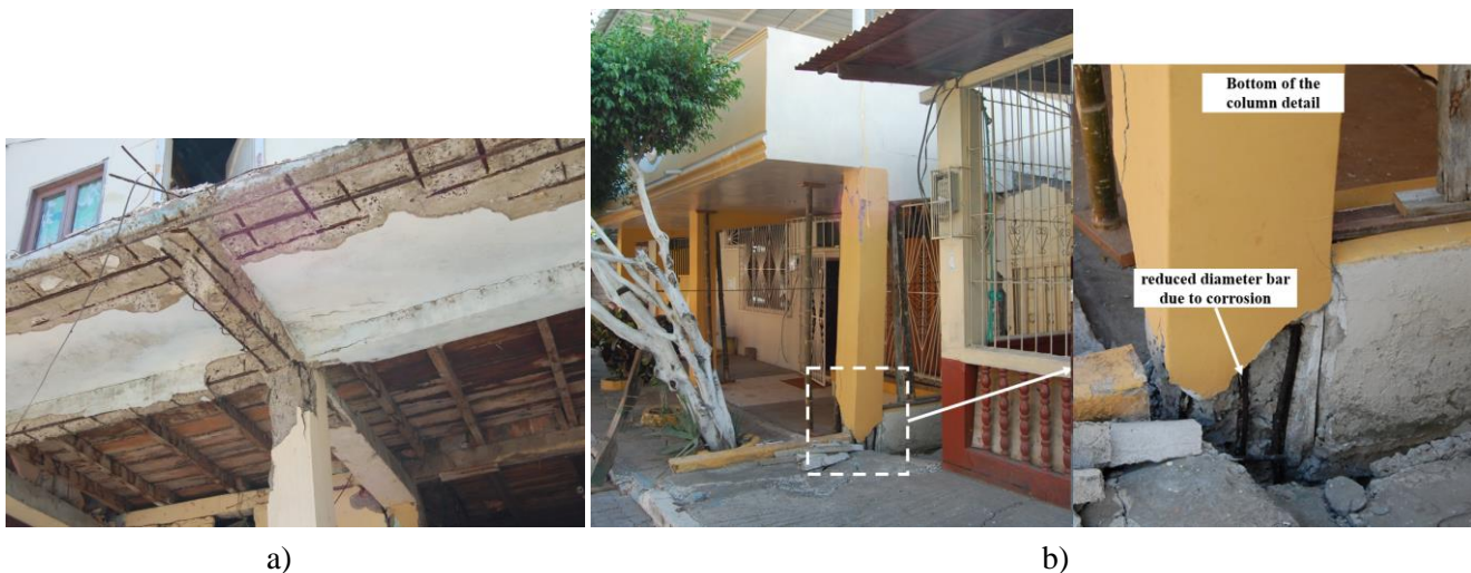
Fig. 13: a) Rebar corrosion in a beam-column connection, and slab reinforcement in a three-story building located in Tarqui, Manta (GPS coordinates: 0°57'7.94"S, 80°42'41.90"W). b) Rebar area reduction at the base of a column and failure due to soil liquefaction in a two-story house located in Tarqui, Manta (GPS coordinates: 0°57'19.77"S, 80°42'40.68"W). (Photos by C. Arteta Torrents)
