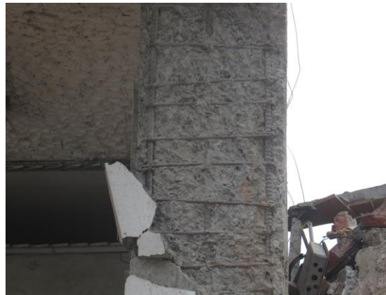
Fig. 8: Column with spalled-off concrete cover and evidence of healthy a core thanks to closely spaced perimeter hoops and cross-ties. Zona Cero in Portoviejo. (GPS coordinates: 1°3'13.53"S, 80°27'8.60"W) (Photo by E. Miranda)
