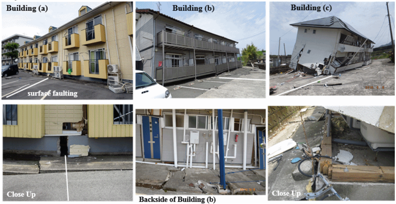
(a) An old steel apartment on the surface fault (Damage grade 4) (b) An old wooden apartment on the surface fault (Damage grade 4) (c) An old wooden apartment on the surface Fault (Damage grade 5)
