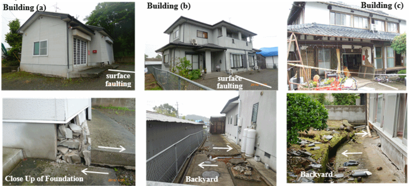
(a) An old wooden house on the surface fault (Damage grade 4) (b) A new house on the surface fault (Damage grade 1) (c) A very old wooden house on the surface fault (Damage grade 4)
