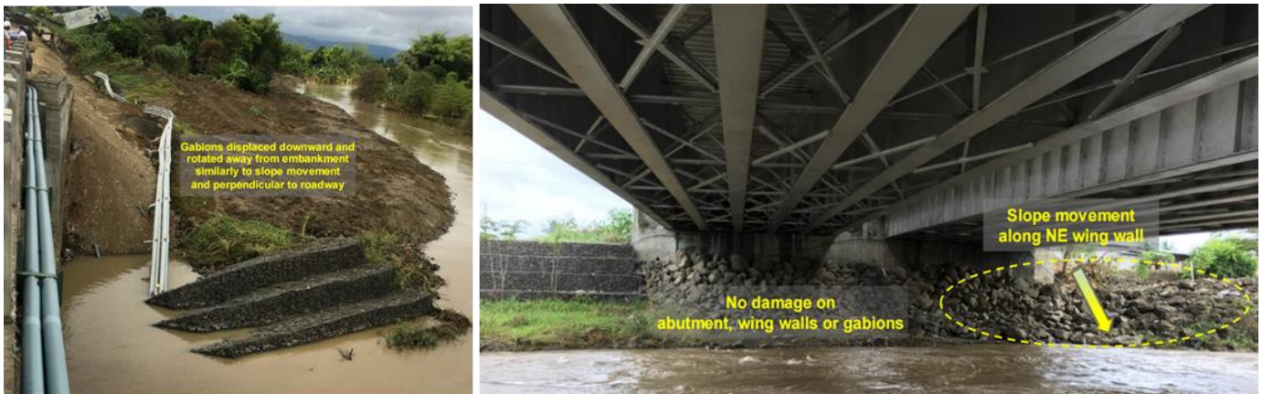
Figure 16. Mejia Bridge. Left: Failures of SW abutment and gabions (GPS: 0°59'23.5"S, 80°28'11.6"W). Right: North abutment performance (GPS: 0°59'24.94"S, 80°28'11.26"W). For details see [1].
