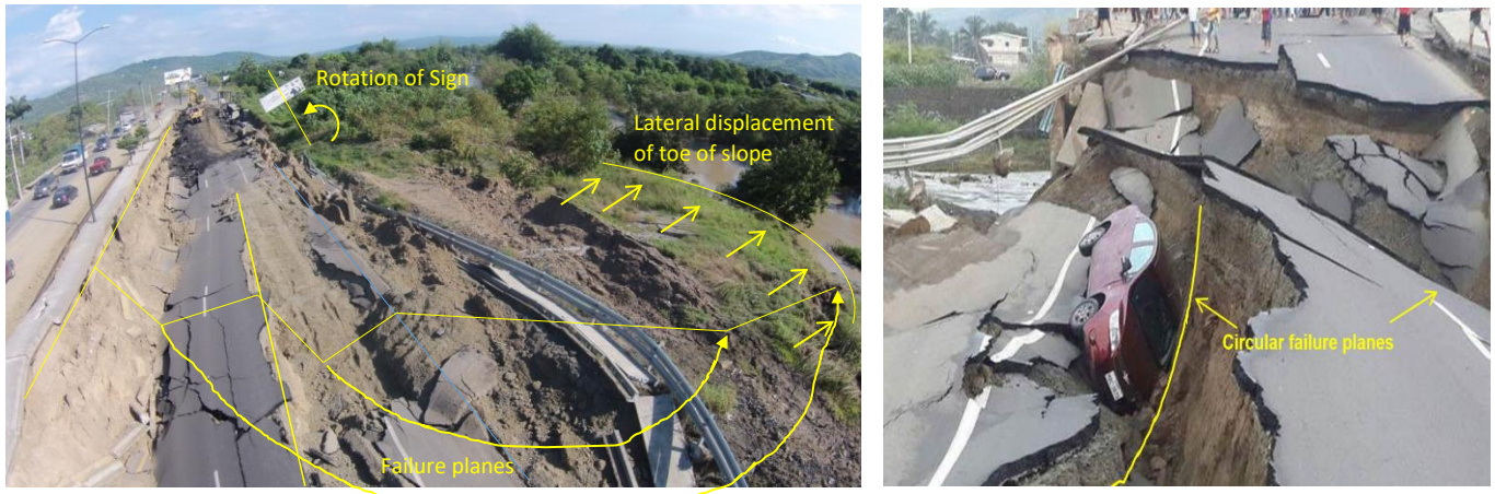
Figure 15. Mejia Bridge. Right: Aerial view of embankment failure with assumed movement and failure modes marked with yellow (after COE-3, GPS: 0°59'24"S, 80°28'11"W). Left: Embankment view after earthquake. For details see [1].
