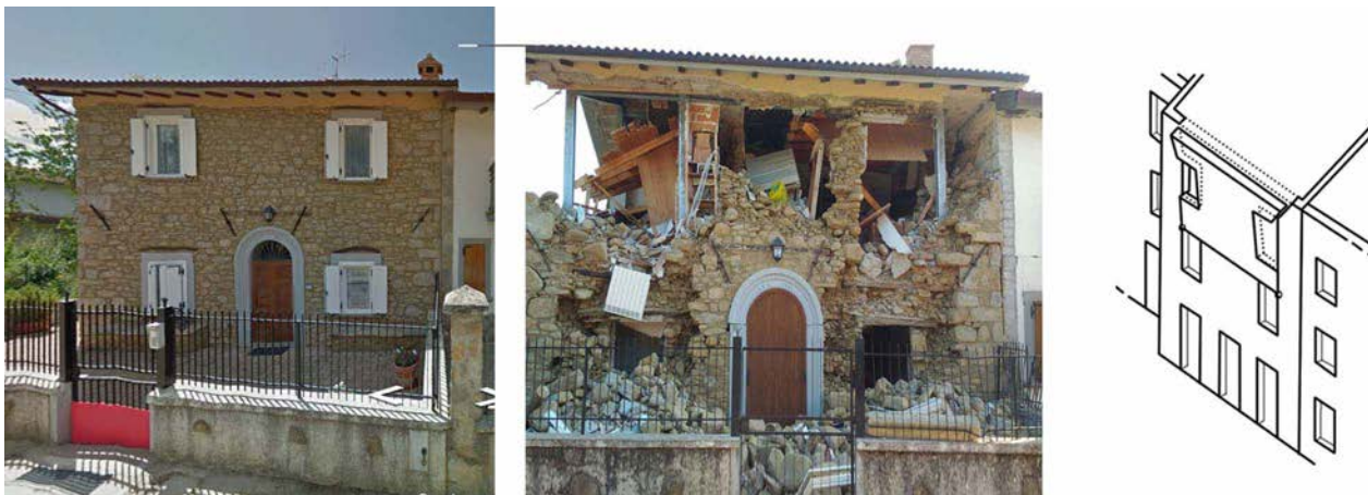
Fig. 4h- Example of masonry building with inadequate interventions of consolidation. Steel elements, at the second floor, hammered the rubble masonry wall determining the overturning of the all upper part of façade. The presence of ties has limited the collapse at the lower part of the façade, Rocchetta village
