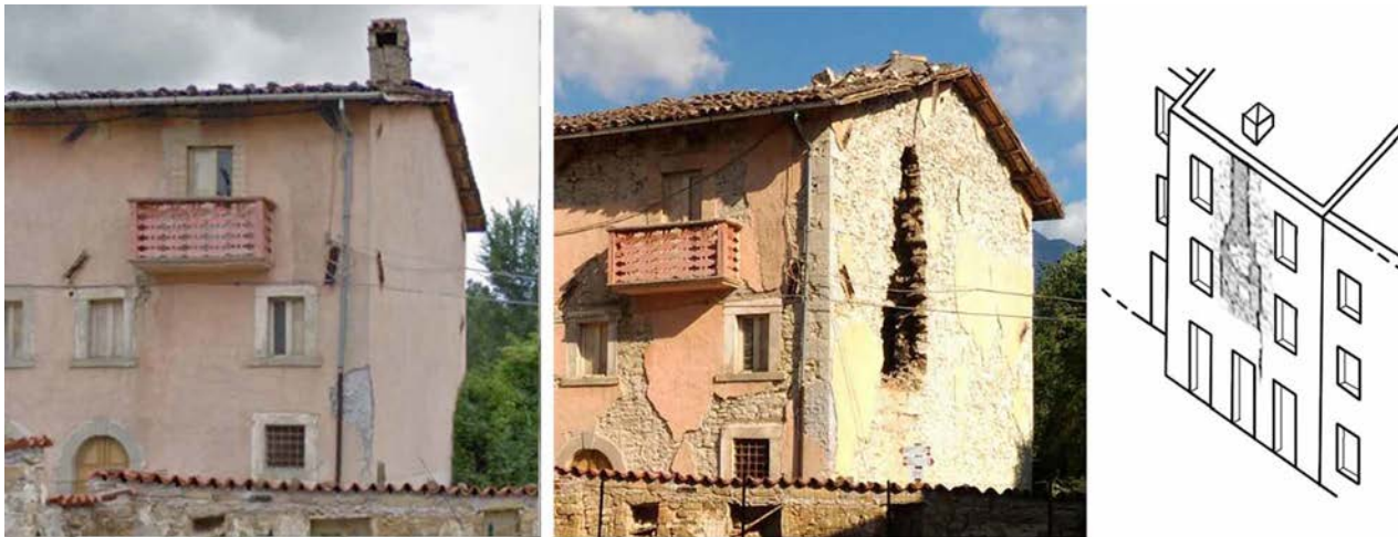
Fig. 4a- Out-of-plane mechanism due to material irregularity and local weakness of masonry wall determinate by the presence of a flue, Cascello village
