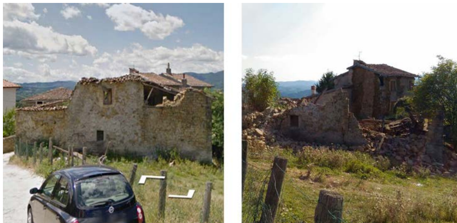
Fig.2a - An abandoned building collapsed by disaggregation. The total absence of maintenance has exposed the interiors to atmospheric agents, causing an important deterioration of the masonry made of pebbles and mud mortar, Casale village
