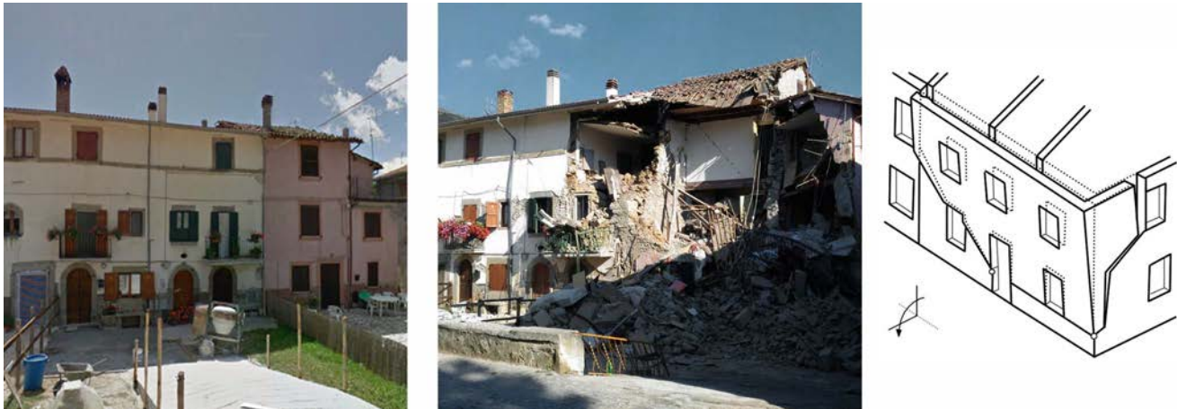
Fig. 4g - Composite overturning of the façade in the terraced aggregate, San Lorenzo a Flaviano
