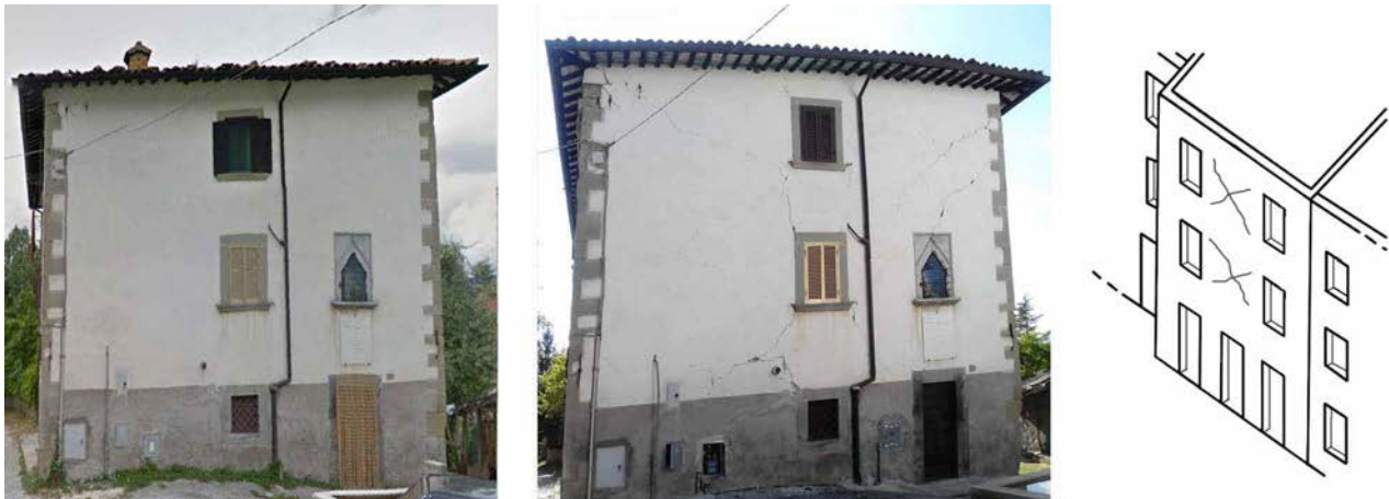
Fig. 5c – The isolated building shows both diagonal and vertical cracks; it exhibits tie-rods just at the second floor and corners bonds with regular and squared medium size blocks, Sommati village
