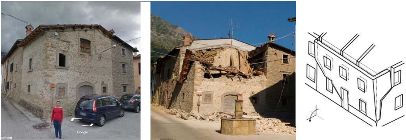
Fig. 4f – Composite overturning mechanism of façade due to the absence adequate quoins between the additions, to the presence of a big opening and of other opening in proximity of wall extremity, Cascello village
