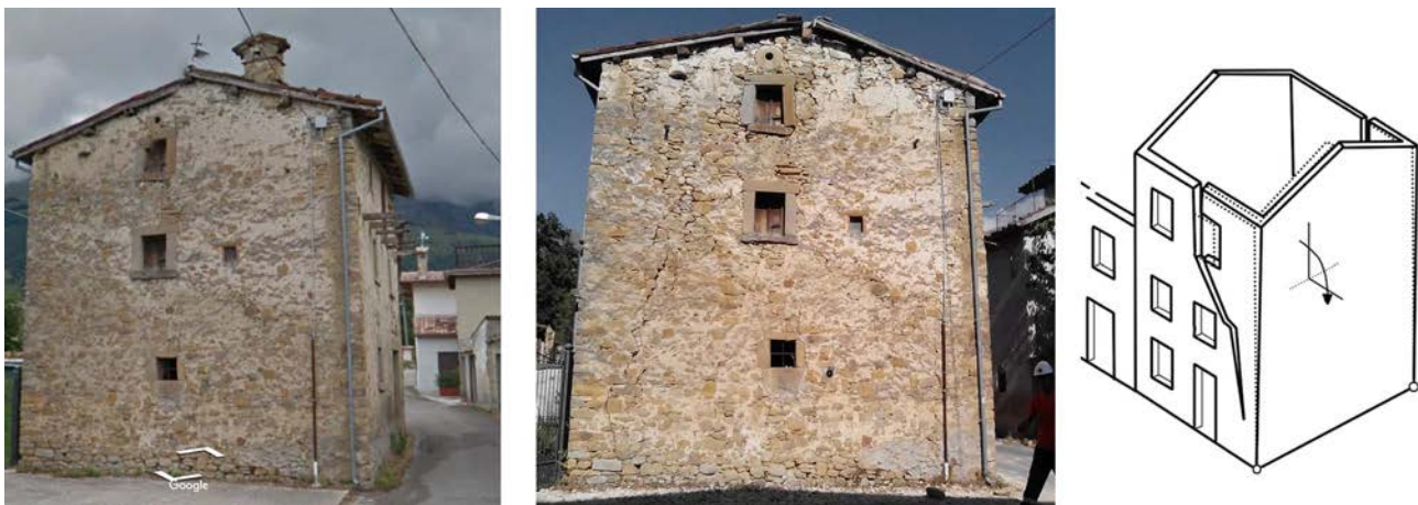
Fig. 5a - The isolated building shows the partial activation of façade overturning which doesn't collapse because of the presence of a tie-rod, located at the second floor. Prato village
