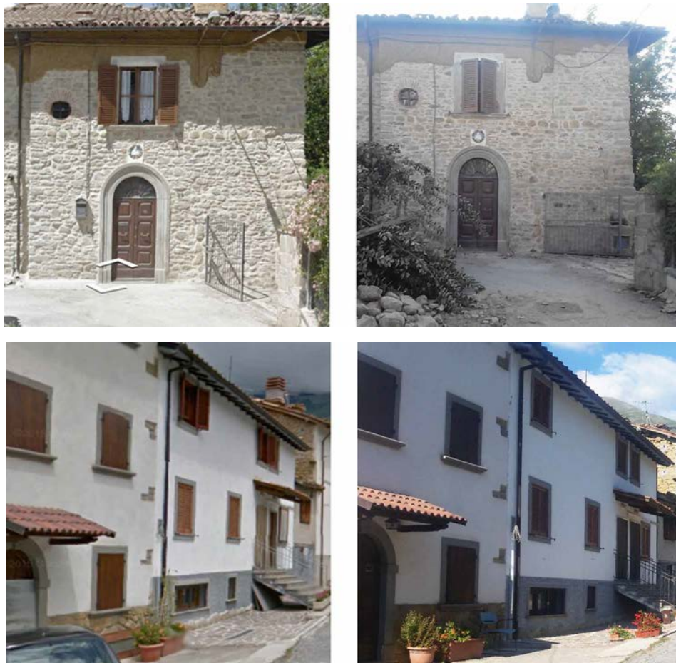
Fig.6a, b - Terraced houses and isolated house with non-structural damage, Sommati and Faizzone villages
