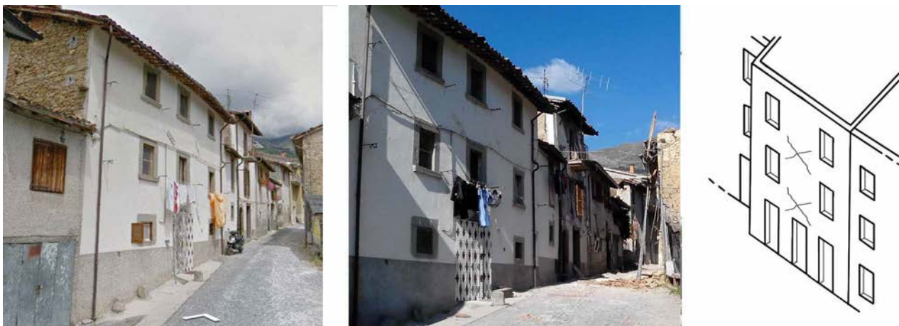
Fig. 5b - The terraced buildings show a good box-behavior characterized by diagonal shear cracks in upper level storey, mainly due to the ties at two levels (second and third floor), Sommati village
