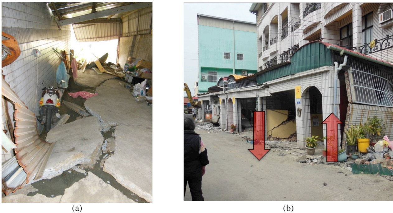
Fig. 11 – Examples of single story additions, lacking interconnected footings with the primary structure: (a) Annan site and (b) Xinshi site (not the structural hinge mechanism that develops within the single story carport beams due to excessive differential settlement of the isolated column footings; the main multi-story structure in the background remained undamaged, whereas the single-story carport was demolished).
