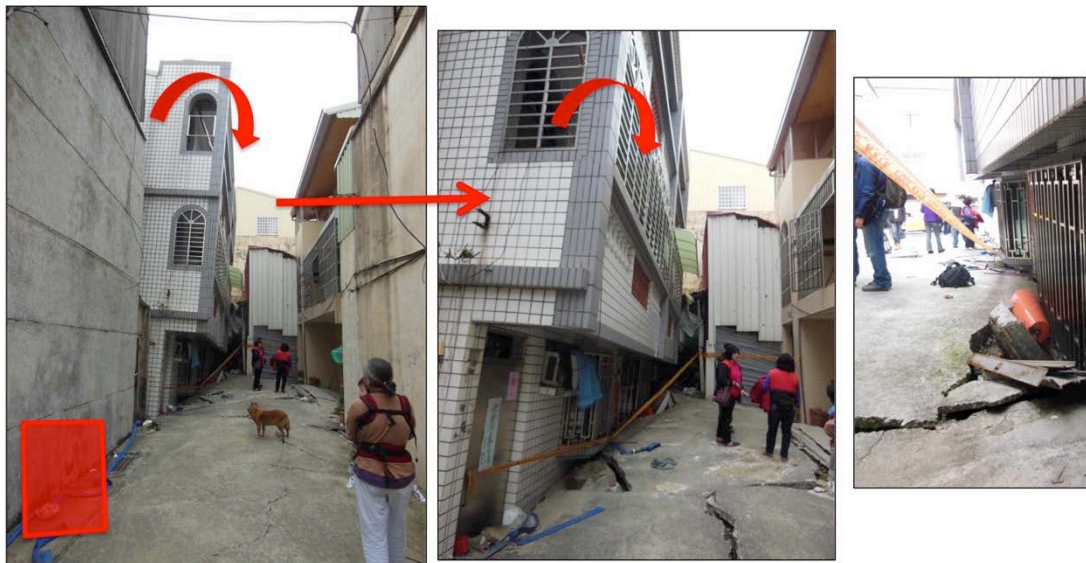
Fig. 10 – Example of mapping worse case ground and structural damage combination (GF3-DF5). (23.0254°, 120.2074°; Lane 161, Hui'an St)
