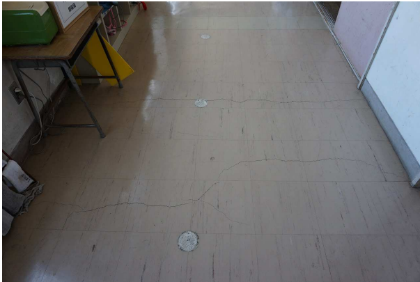
(a) Cracks on floor slabs
