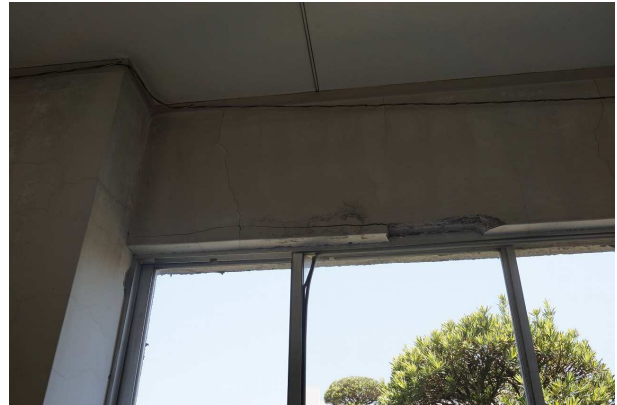
(b) Cracks on beams with hanging walls
