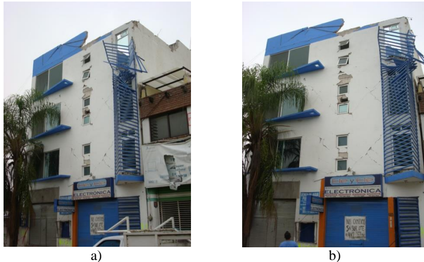
Fig. 13 – Observed damage in an apartment building due to inadequate confinement, located in the Terán neighborhood of Tuxtla Gutiérrez, Chiapas
