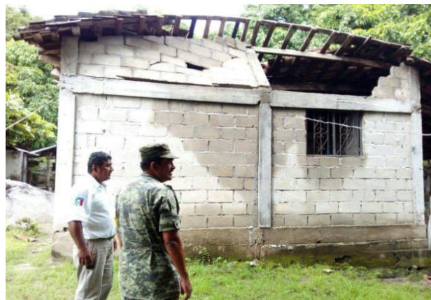
Fig. 7 – Out-of-plane overturning because of inadequate confinement of walls and as a consequence of the lack of lateral support, Pijjiapan, Chiapas
