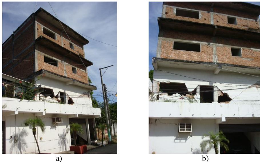
Fig. 15 – Damage to masonry walls in a four-story apartment building in Tonalá, Chiapas
