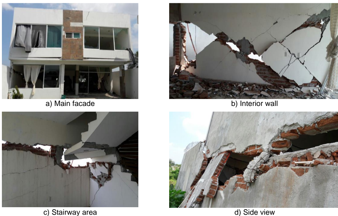
Fig. 12 – Severe structural damage to a residential house located in Tuxtla Gutiérrez, Chiapas (photographs courtesy of BSc. Christian Burguete D'Artote)
