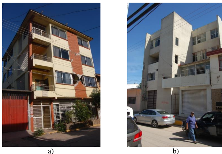
Fig. 14 – Damage to masonry walls of apartment buildings located in Juchitán, Oaxaca
