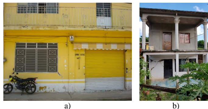
Fig. 9 – Observed damage in poorly confined masonry houses, in Matías Romero, Oaxaca
