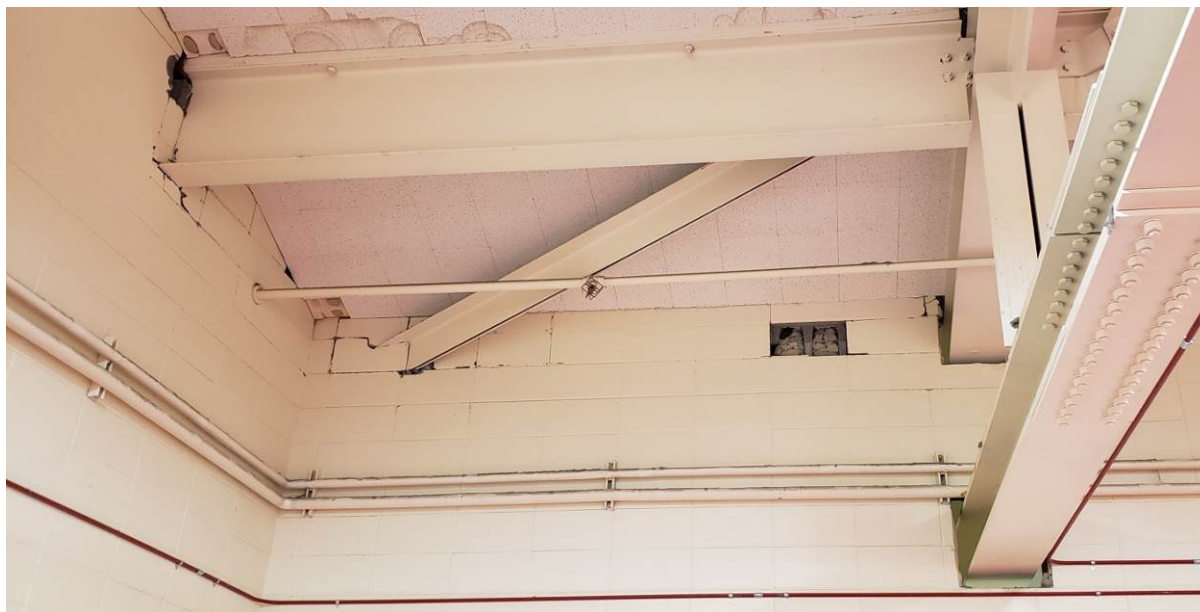
Figure 6 – CMU block at top of wall cracked and loosened due to differential motion of steel roof framing, Houston Middle School. Loose blocks pose a falling hazard to those below. Photo: MSBSD
