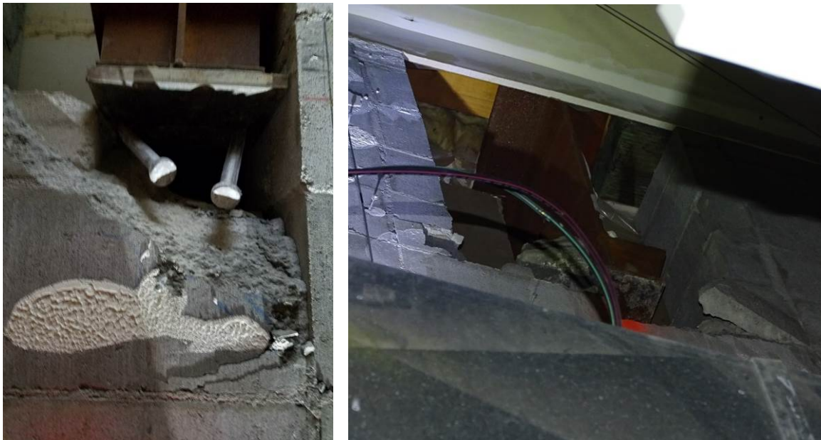
Figure 3 – Failed connection between steel roof girder and CMU wall in second story of classroom wing (left); similar failed connection (right). Photos: Bill Noyes (left), Janise Rodgers (right).
