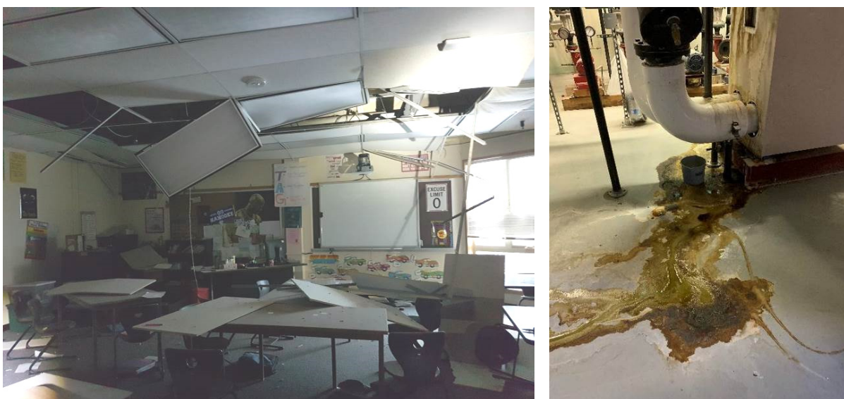
Figure 7 – Example of major ceiling damage, Houston Middle School (left) and glycol leak due to pipe connection damage, Gruening Middle School (right). Photos: MSBSD (left) and Wael Hassan (right)
