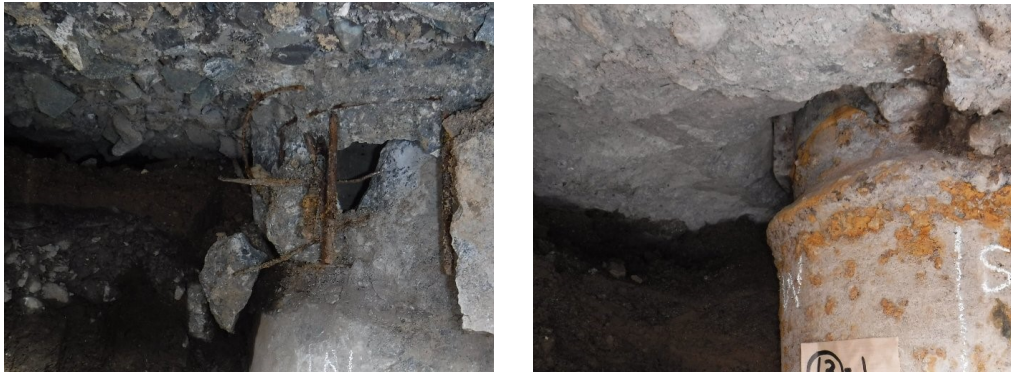
Photo 5 – Failure of precast pretensioned concrete pile and buckling of steel pipe pile
