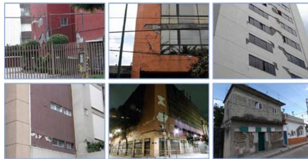
Fig. 8 – Non-structural damage to R/C and mixed type buildings in the affected area due to the September 19, 2017 M 7.1 Puebla-Morelos earthquake. Cracks in the infill walls and detachment of pieces of plaster from the infill walls.
