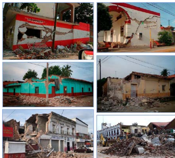
Fig. 14 – Non-structural and structural damage induced by the first earthquake on September 7, 2017 to the adobe and masonry buildings in Oaxaca and Chiapas states.
