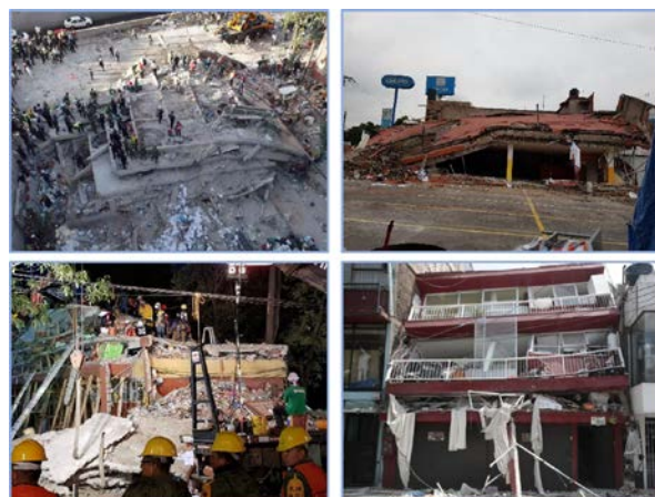
Fig. 11 – Very heavy structural damage (total collapse) of buildings in the Greater Mexico City area induced by the second earthquake in September 2018.
