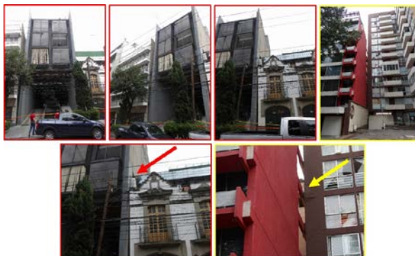
Fig. 13 – Damage induced by pounding between closely spaced buildings due to the September 19, 2017 earthquake.
