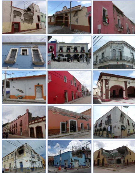
Fig. 15 – Non-structural and structural damage induced by the second earthquake on September 19, 2017 to the adobe and masonry buildings in Puebla and Morelos states.
