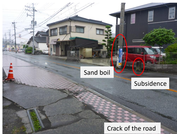
Fig. 1 – Damage caused by liquefaction at Kumato City
