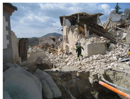
Fig. 4 - All structures in Castelnuovo on a hilltop were totally or partially collapsed (from GEER 2009,[5])
